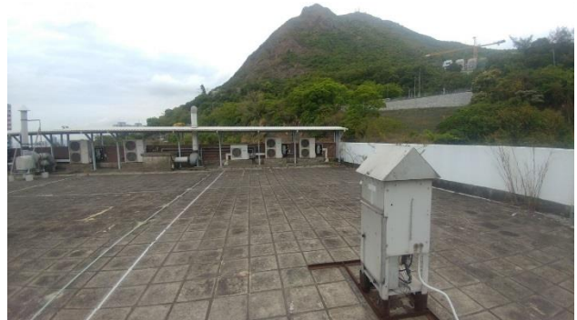
Figure 2 – Location of HVS and the outdoor units of split-type air-conditioners at ID 5
