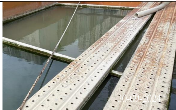
Photo 5 (Water quality of water treatment tank at 6/WSD)
