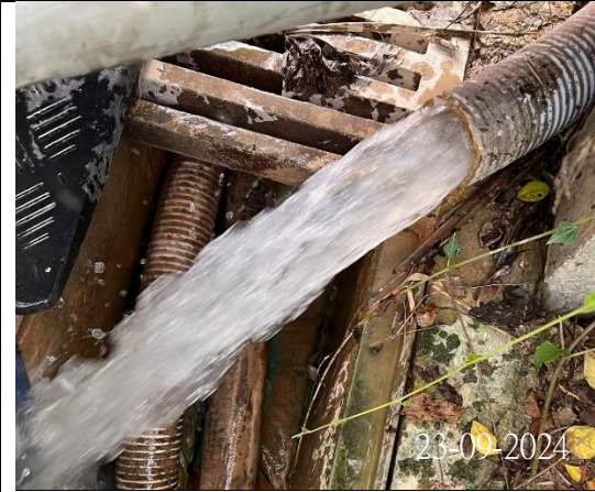
Photo 3 (Discharge point at 6/WSD)
