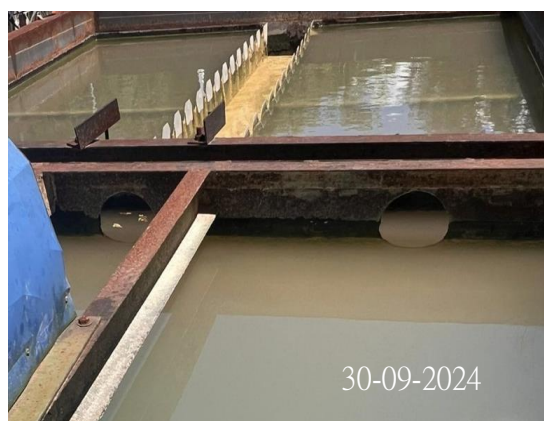
Photo 7 (Water quality of water treatment tank at 1/WSD)
