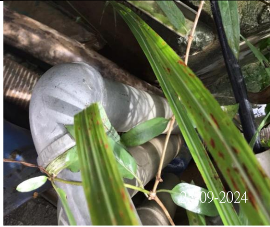
Photo 3 (Discharge point at 6/WSD)
