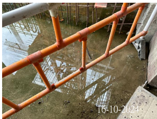
Photo 5 (Water accumulation on the site area at 6/WSD)
