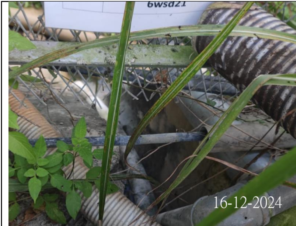
Photo 3 (Discharge point at 6/WSD)
