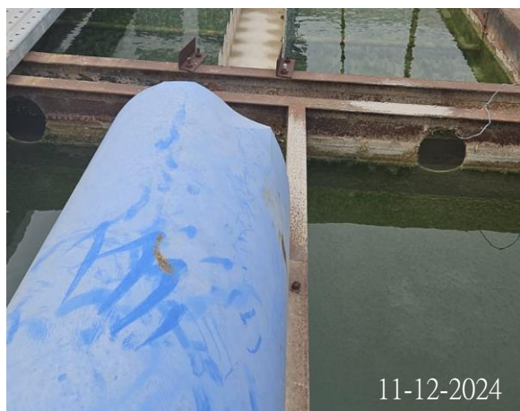
Photo 5 (Water quality of water treatment tank at 1/WSD)
