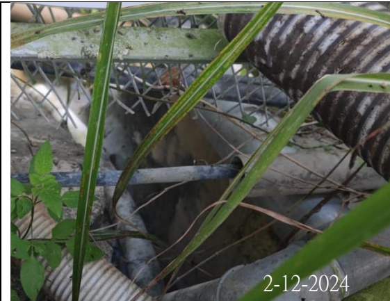
Photo 3 (Discharge point at 6/WSD)
