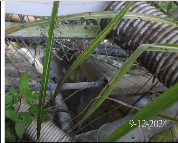
Photo 3 (Discharge point at 6/WSD)
