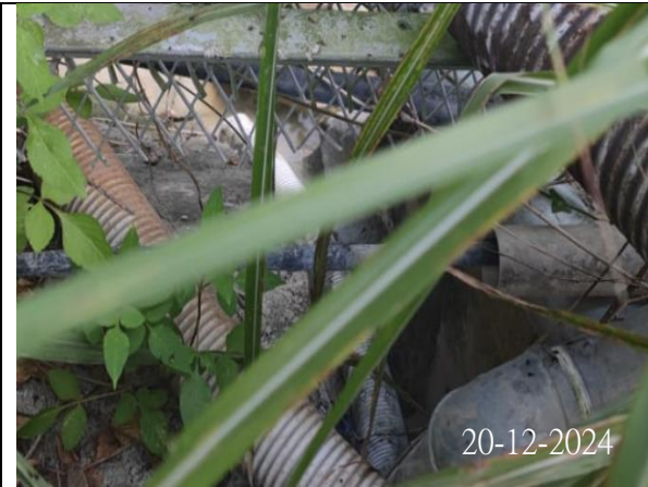
Photo 3 (Discharge point at 6/WSD)
