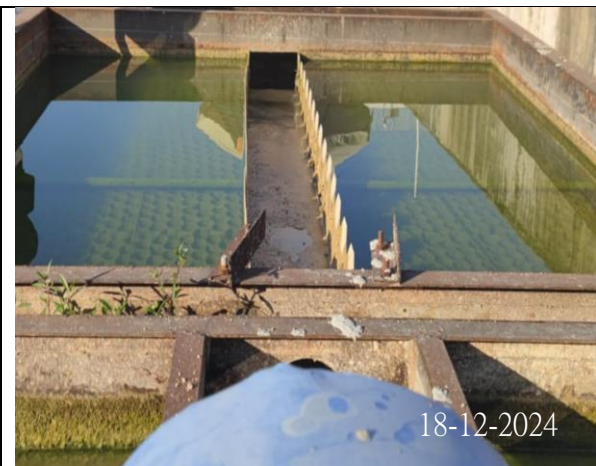
Photo 3 (Water quality of water treatment tank at 6/WSD)
