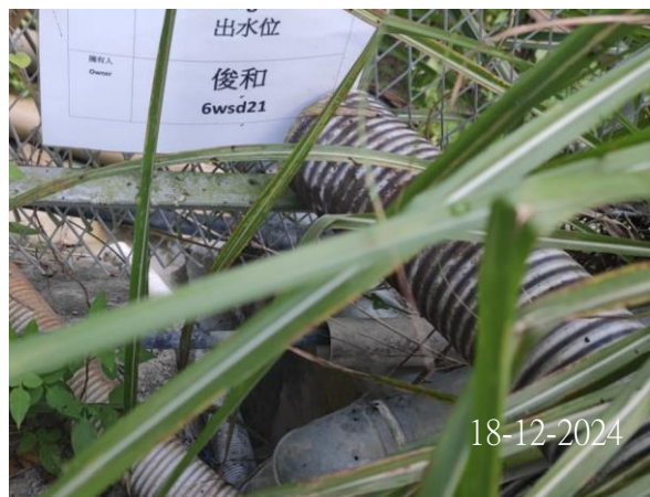
Photo 4 (Discharge point at 6/WSD)
