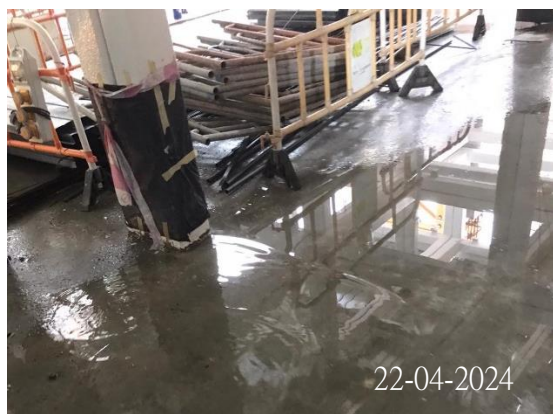
Photo 5 (Water accumulation on the site area at 6/WSD)
