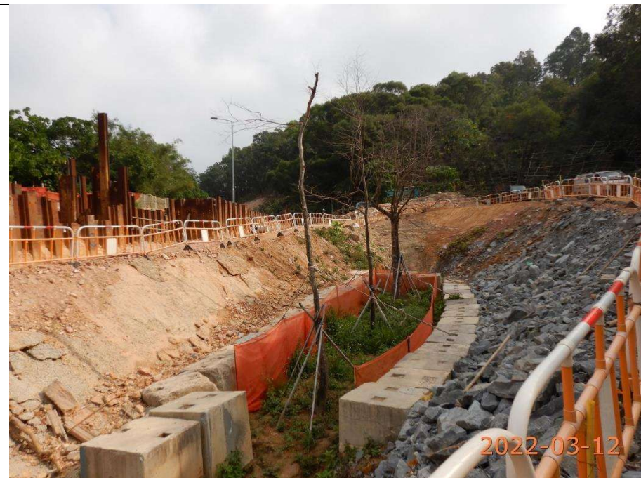
Formation of ditch to guide surface runoff to water pumping location, moist soil surface observed
