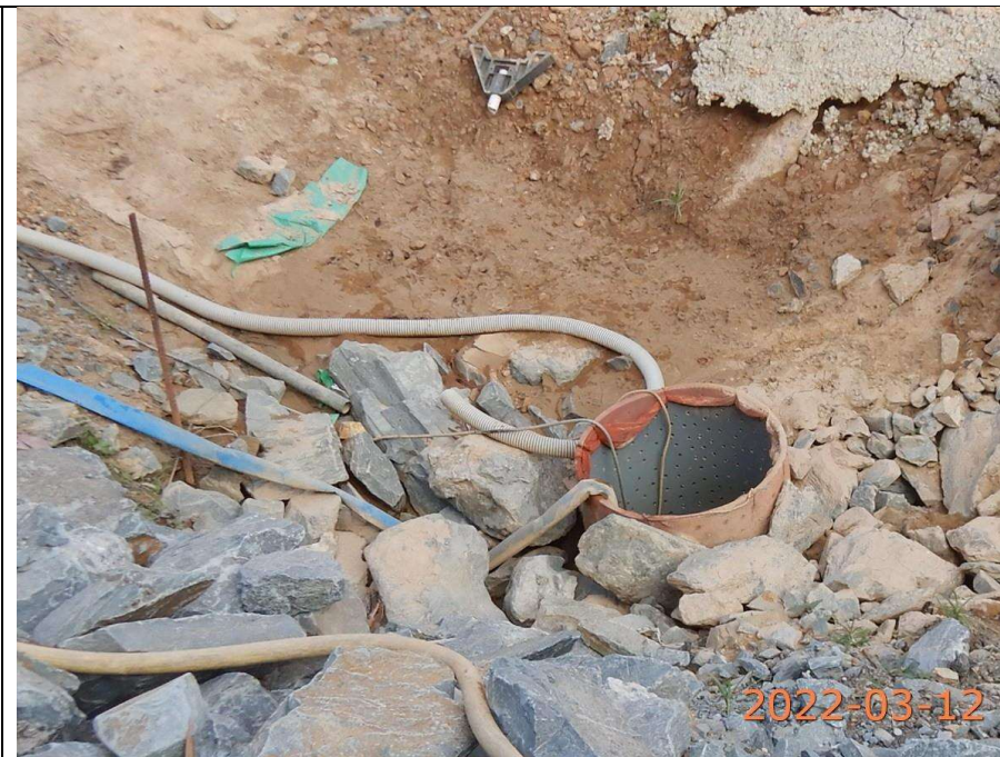
Submersible pump standby
