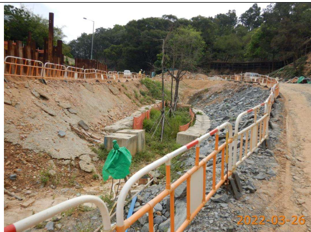
Formation of ditch to guide surface runoff to water pumping location, dewatering was carried out during rainy days
