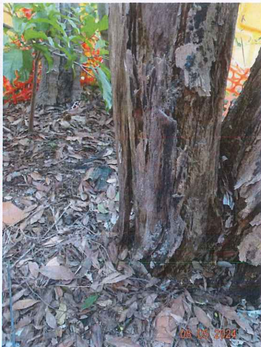
12: U041_Another crack enlarged on May 2024_Close up
