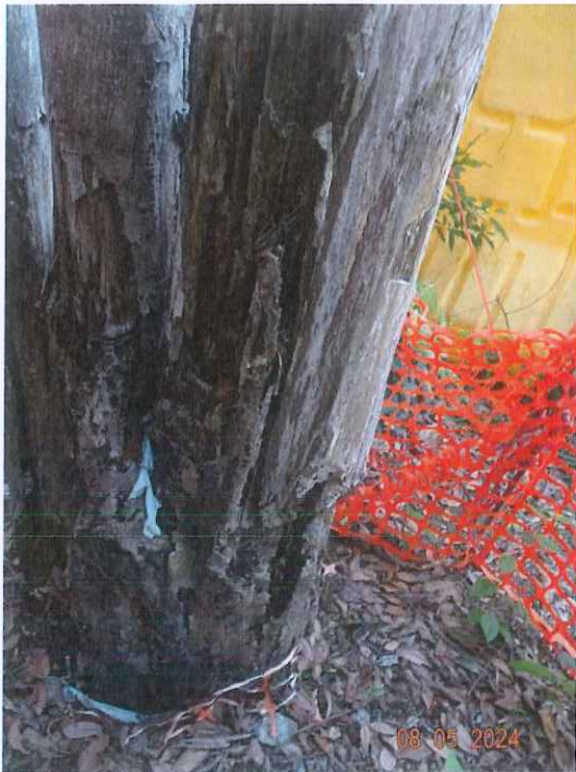
9: U041_Dead stump_Close up, crack enlarged since late March 2024, extra staking was provided on 21 March 2024
