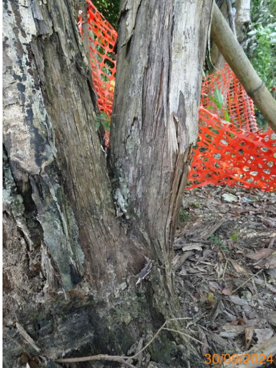
9: U041_Crack on trunk
