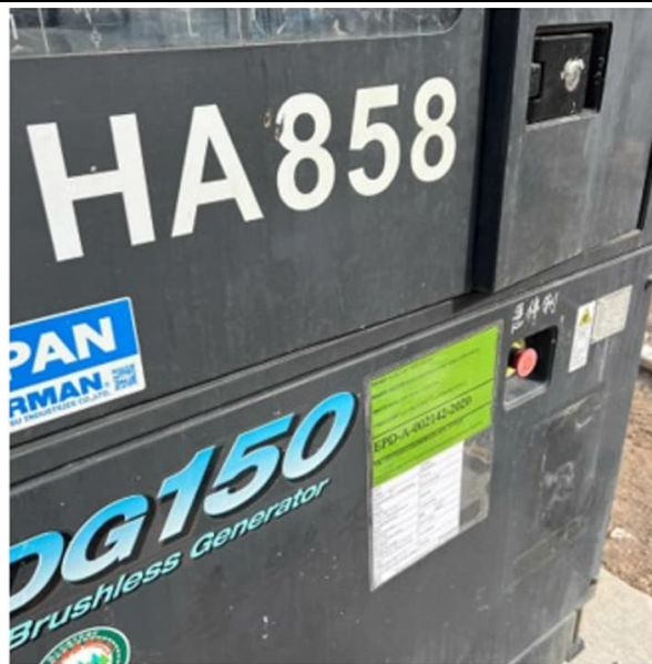
Photo 2: Power Mechanical Equipment with Quality Power Mechanical Equipment (QPME) labels were used at site to lower the noise nuisance to the nearby residents.
