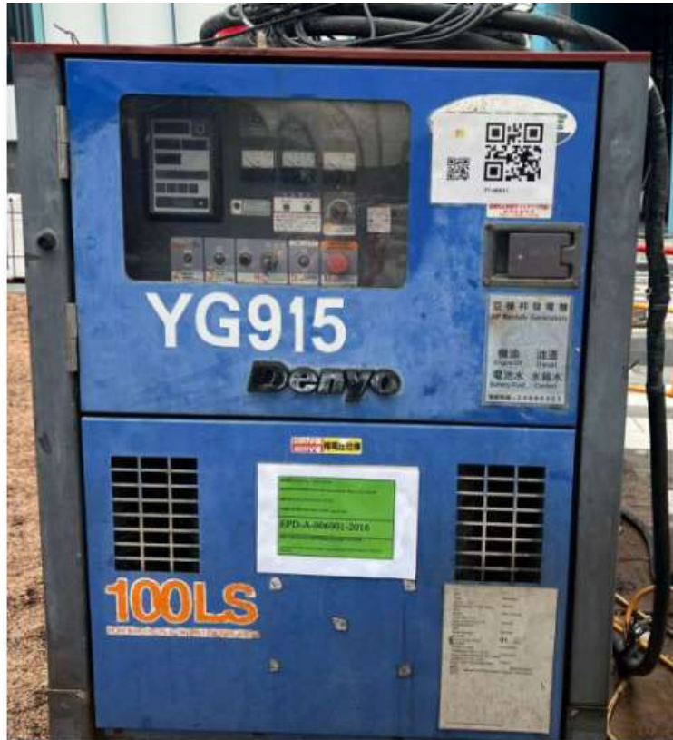
Photo 2: Power Mechanical Equipment with Quality Power Mechanical Equipment (QPME) labels were used at site to lower the noise nuisance to the nearby residents.
