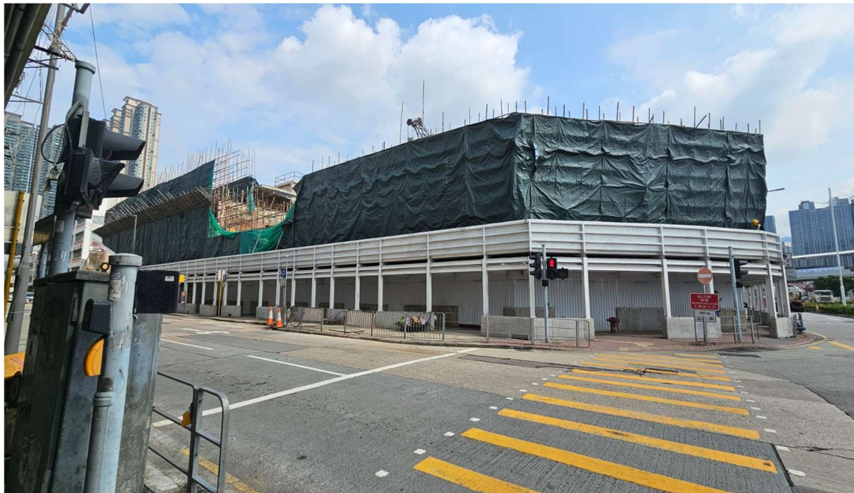
Photo 1a and 1b: Nearby demolition work at The Hong Kong Society for the Blind Workshop and Hostel on 29 August 2024.
