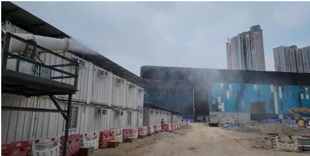
Photo 4: Water misting cannon has been provided for dust suppression on site.
