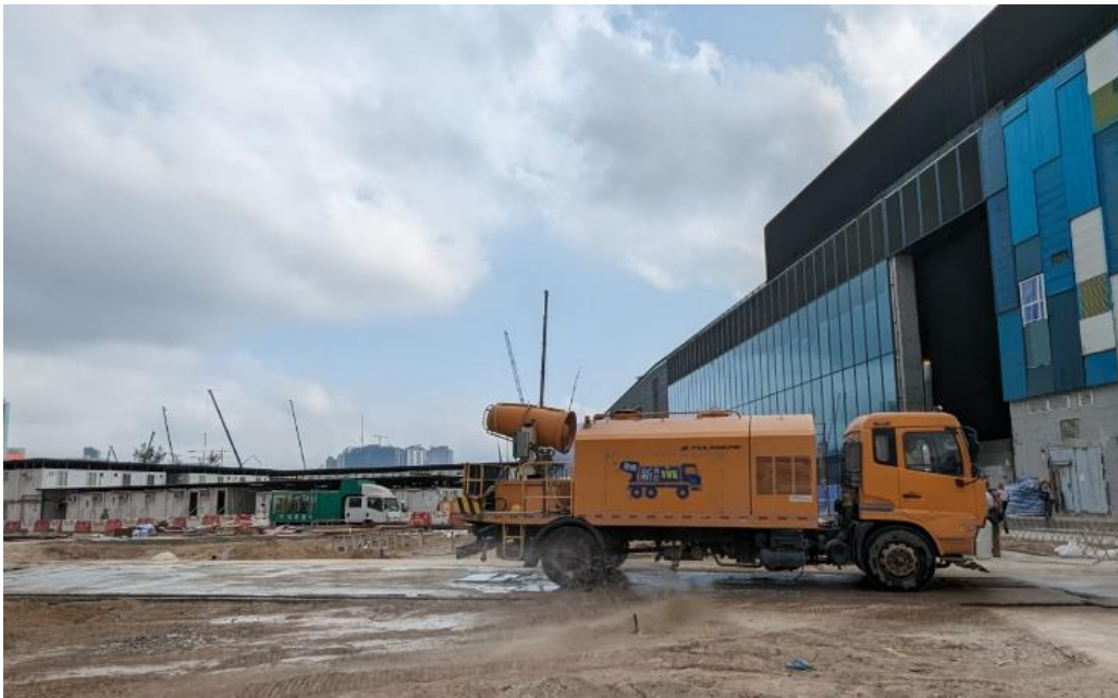
Photo 3: Water spraying truck has been provided on haul road to maintain wet surface.
