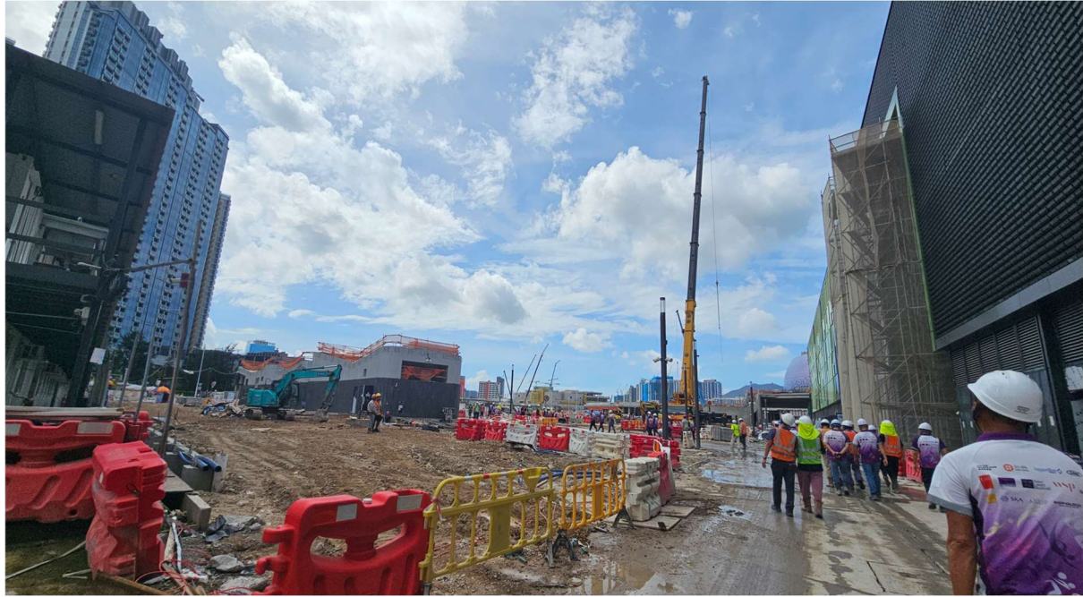
Photo 1: Regular site inspection carried out for checking dust mitigation measure on site. (25 June 2024)
