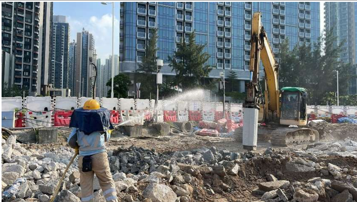
Photo 3: Noise acoustic wrapping has been provided for the breaker to reduce noise emission from the breaking work.
