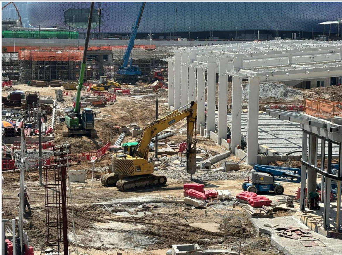
Photo 1a and 1b: Ground breaking work was observed within Kai Tak Sports Park area on 26 September 2024.
