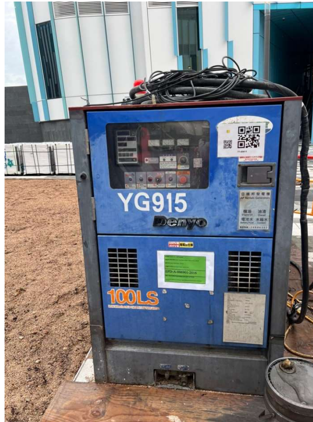
Photo 2: Power Mechanical Equipment with Quality Power Mechanical Equipment (QPME) labels were used at site to lower the noise nuisance to the nearby residents.
