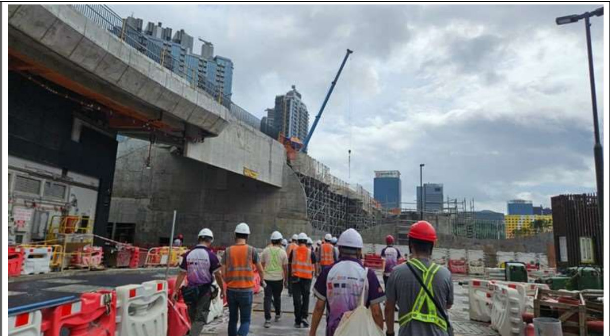
Photo 4: Regular site inspection was carried out to audit the implementation of mitigation measures on site.
