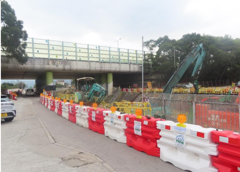
Photo 11: Construction works inside Yuen Long Town Nullah (Section 2) by the other Contractor
