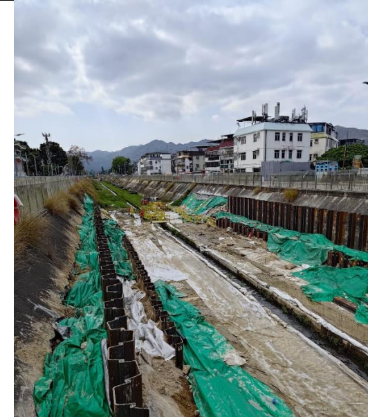
Photo 12: Construction works inside Yuen Long Town Nullah (Section 1) by the other Contractor
