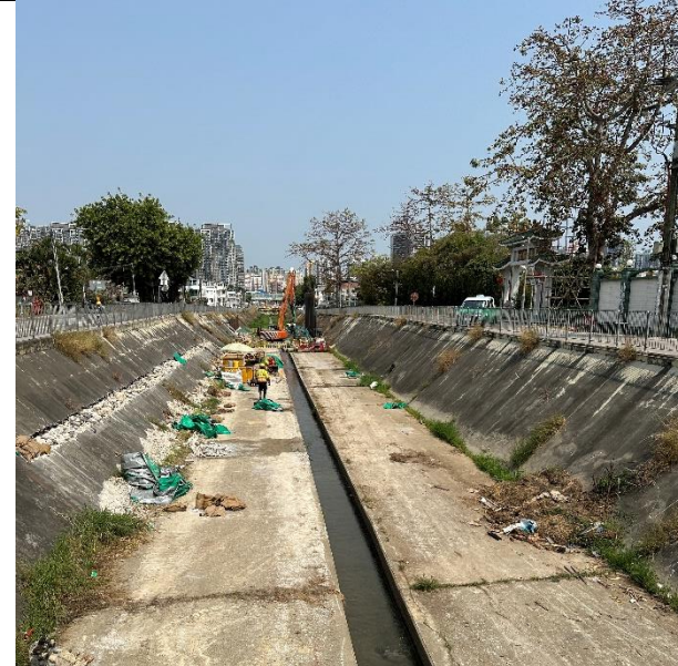
Photo 12: Construction works inside Yuen Long Town Nullah (Section 1) by the other Contractor
