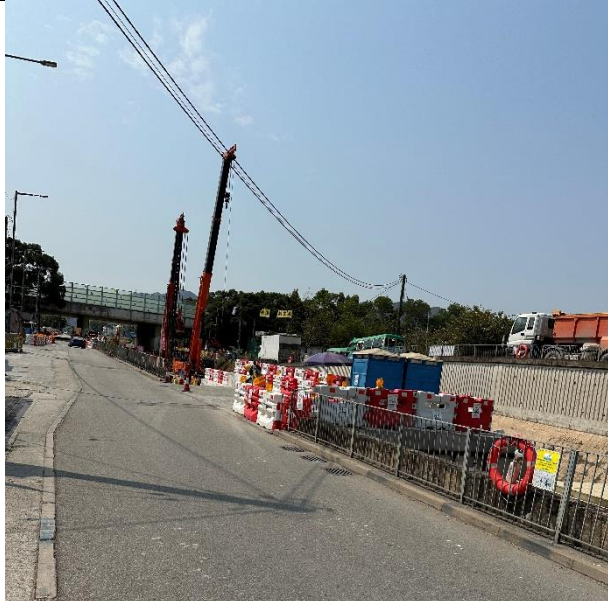
Photo 11: Construction works inside Yuen Long Town Nullah (Section 2) by the other Contractor
