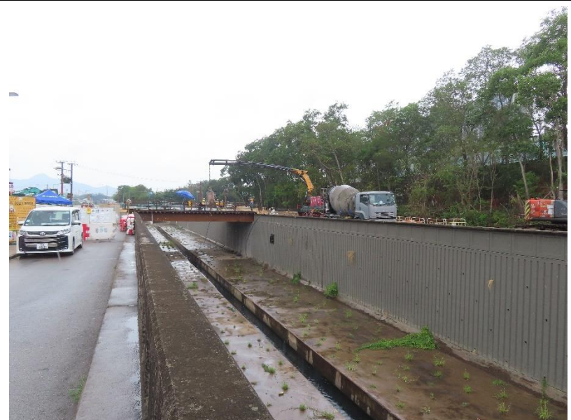
Photo 12: Construction works inside Yuen Long Town Nullah (Section 1) by the other Contractor
