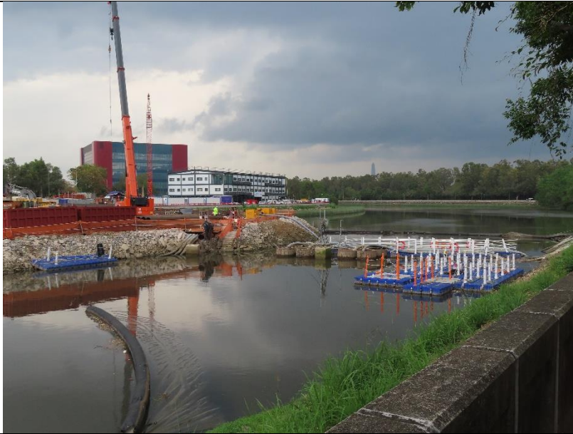
Photo 9: Sheet piling cofferdam construction at section 4 of the Yuen Long Town Nullah
