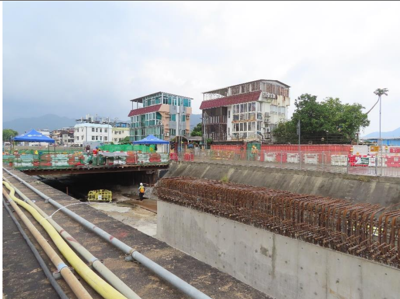
Photo 11: Construction works inside Yuen Long Town Nullah (Section 1) by the other Contractor
