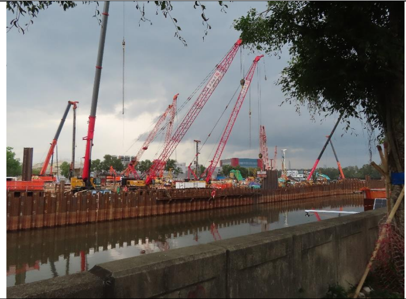
Photo 10: Sheet piling cofferdam construction at section 4 of the Yuen Long Town Nullah
