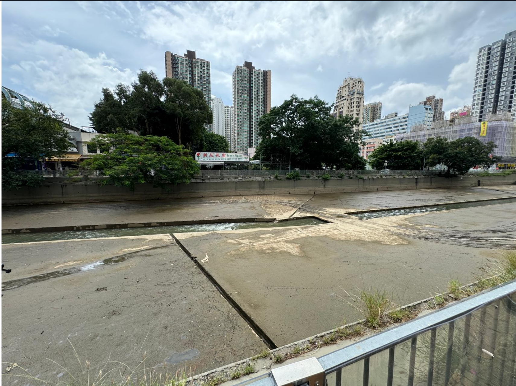
Photo 4 – Mud and sediment in the nullah near OP6 (Taken on 18 June 2024)
