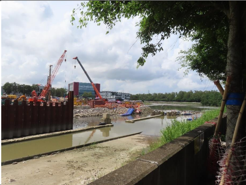
Photo 4: Sheet piling cofferdam construction at section 4 of the Yuen Long Town Nullah
