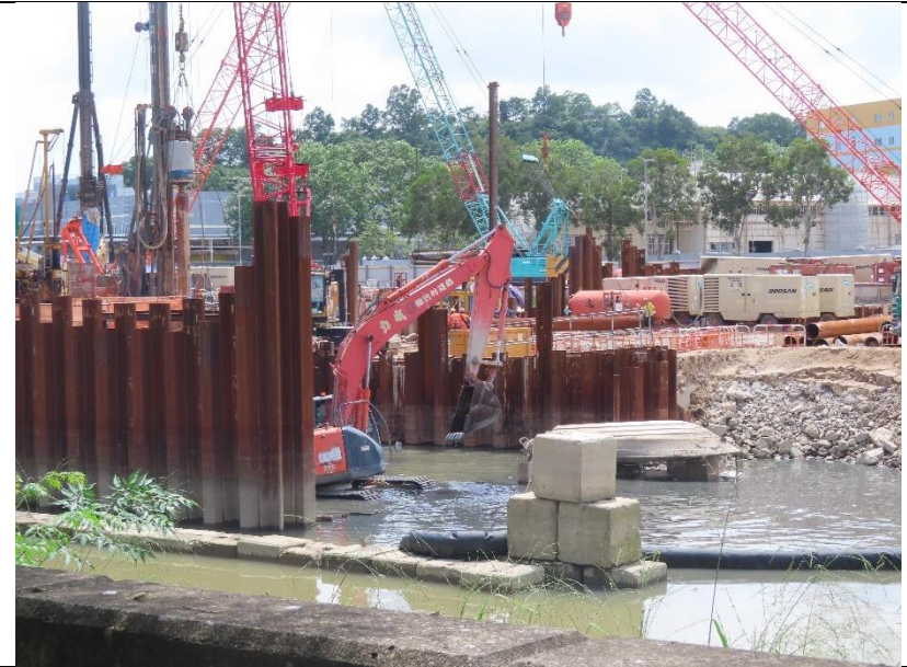
Photo 5: Sheet piling cofferdam construction at section 4 of the Yuen Long Town Nullah
