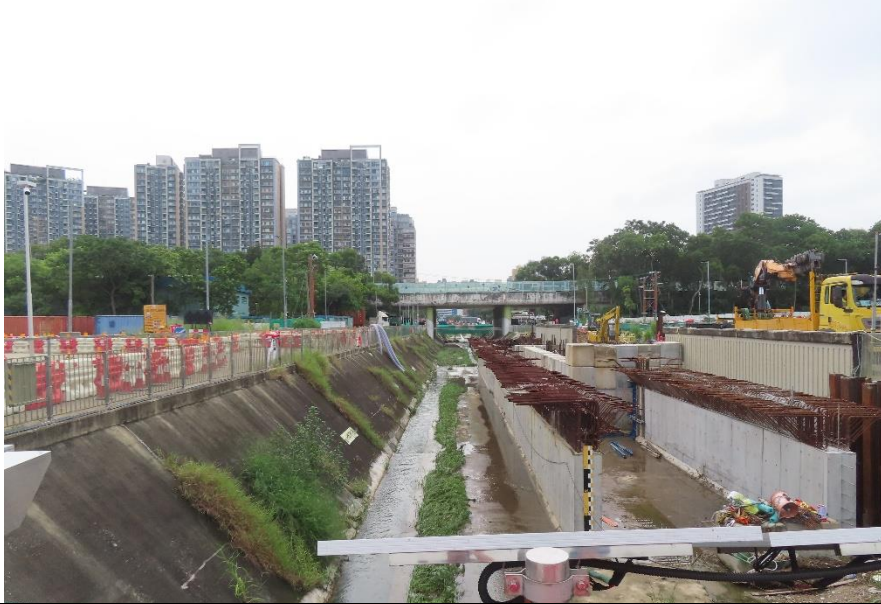
Photo 5: Existing intersection of YLN & YLBF refinements at section 1 of the Yuen Long Town Nullah
