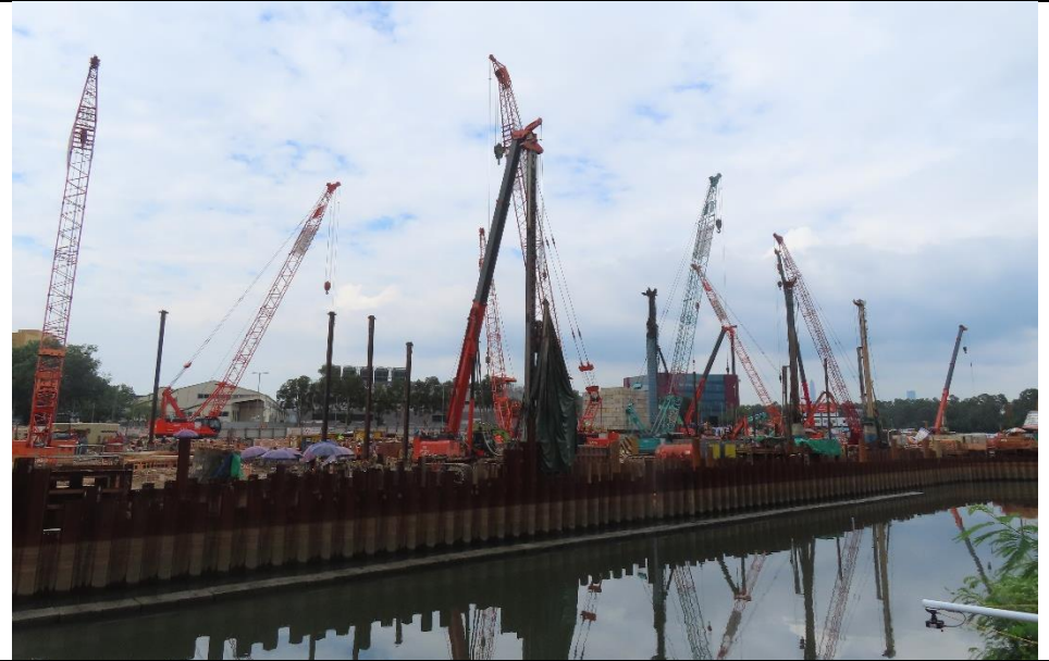
Photo 6: Sheet piling cofferdam construction at section 4 of the Yuen Long Town Nullah
