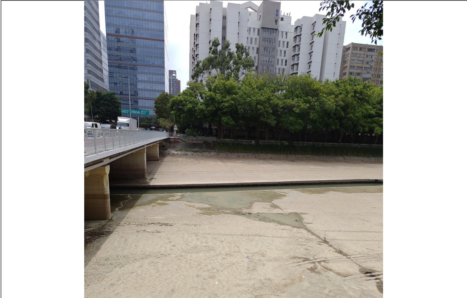
Photo 2 – Sediment on the nullah area between OP2 and OP4 (Photo taken on 12 September 2024)
