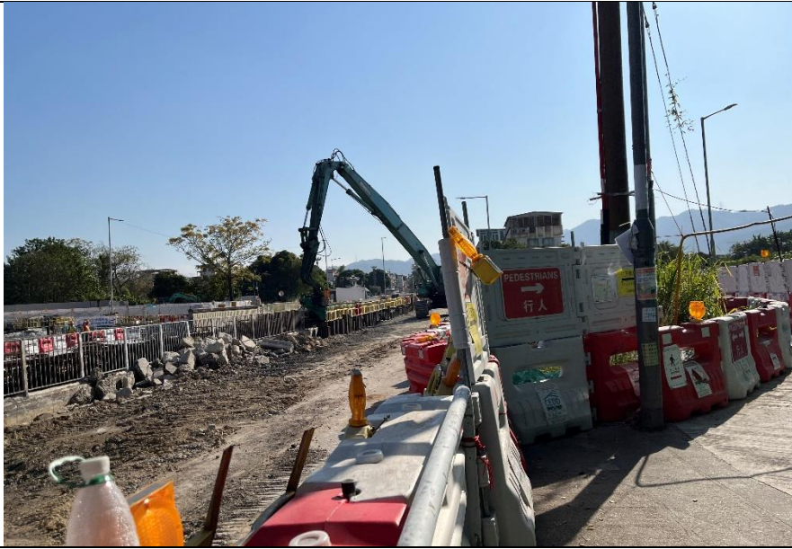
Photo 5: Existing intersection of YLN & YLBF refinements at section 1 of the Yuen Long Town Nullah
