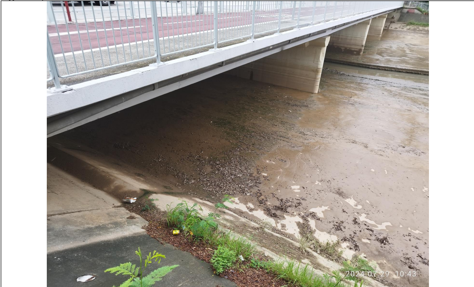
Photo 1 – Sediment remaining in the nullah (Taken on 29 July 2024)
