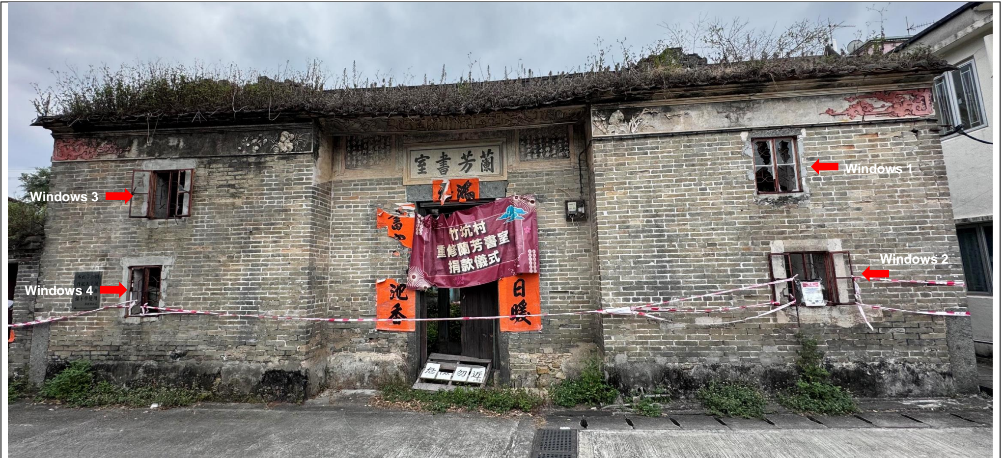
G2.1 W Elevation – General View of Study Hall (Front door, Windows 1, Windows 2, Windows 3 and Windows 4)
