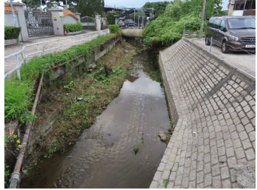
Proposed Drainage Works Area of Lin Fa Tei (Downstream) (CH.A 818.86 ~ CH.A 500.00) Date taken: 22 nd November 2023
