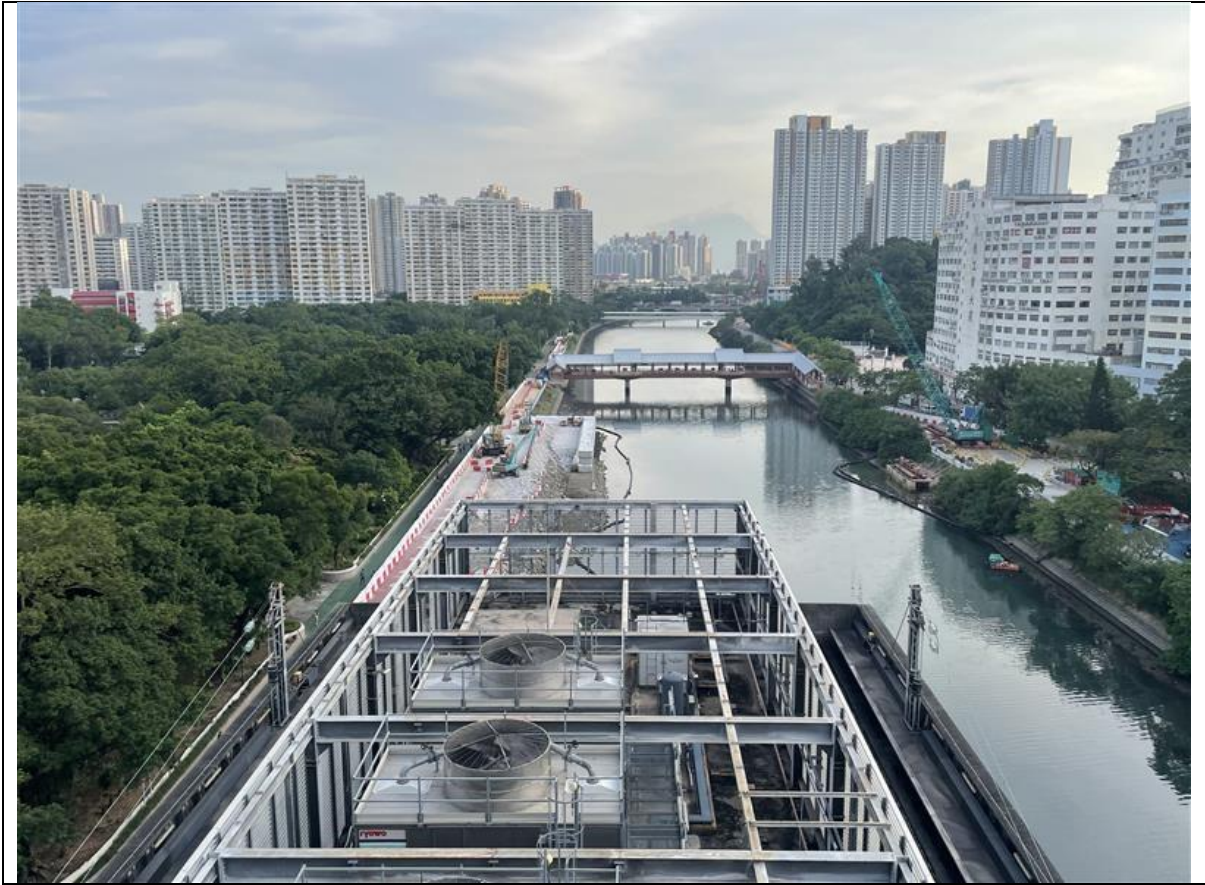
Site preparation works along Tuen Mun River Channel and construction of temporary platform
