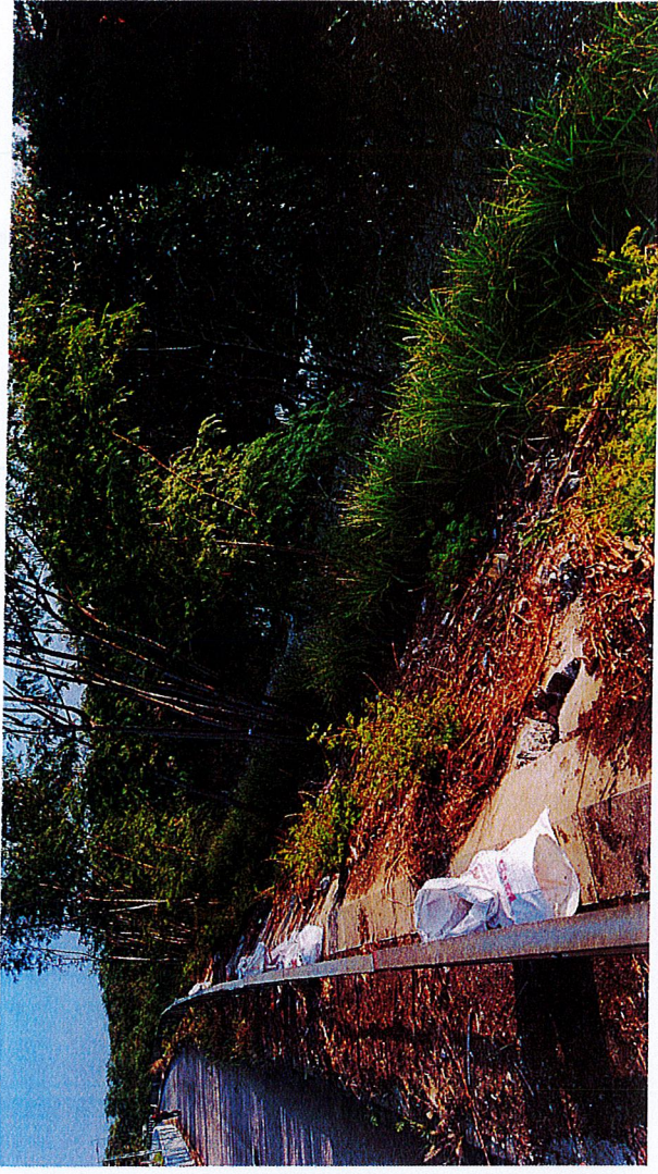
The slope surface of the riverbank is protected by a concrete slab.
