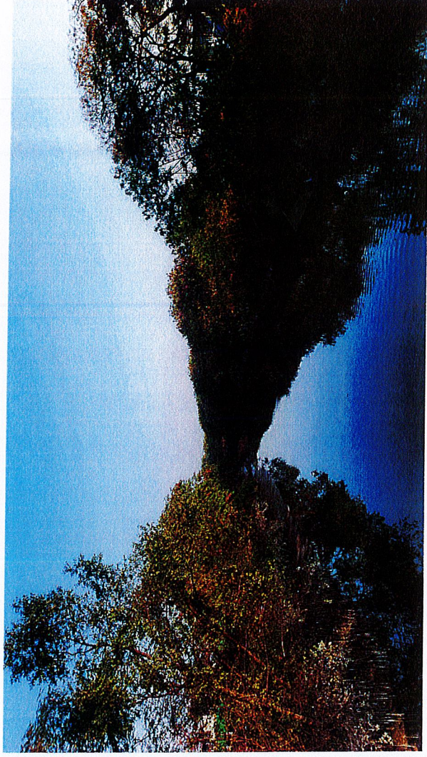
Drainage channel with sloped riverbank at 30 degree or steeper on both sides
