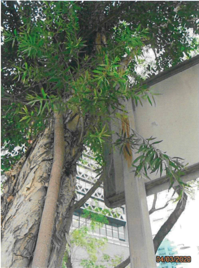
0004 - Conflict with road sign
