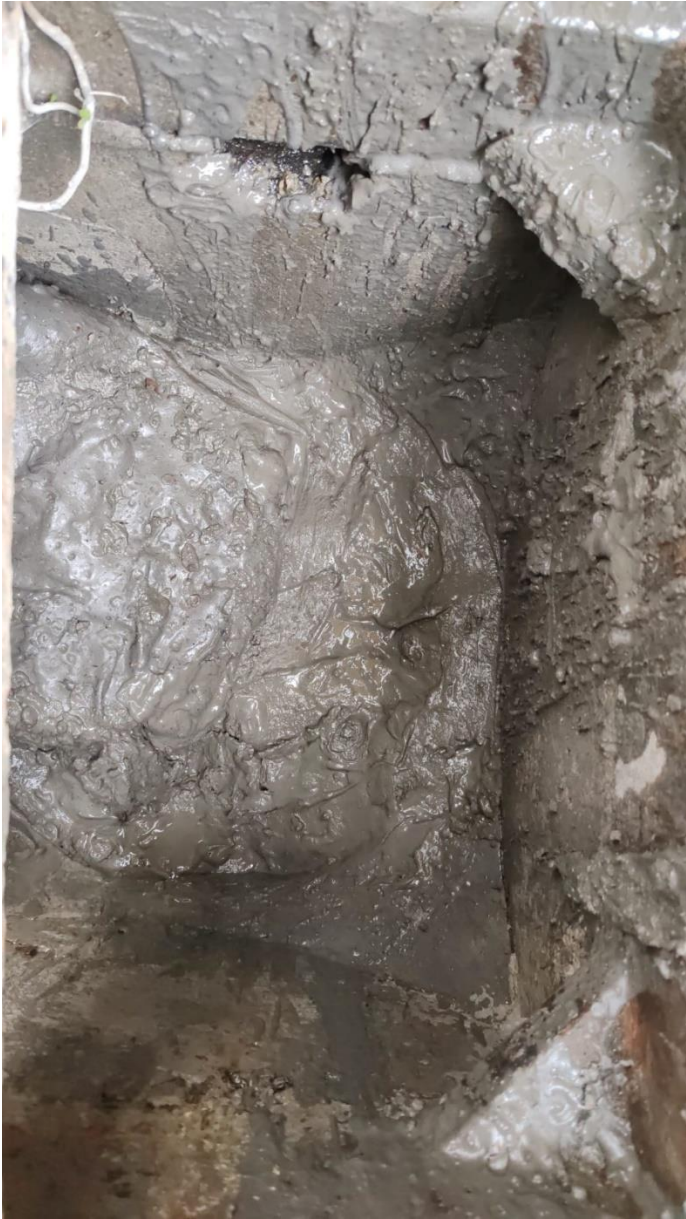
Remark 2: Site photo of the roadside gullies
