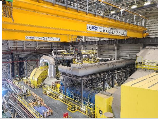
Turbine Hall (Interior)
