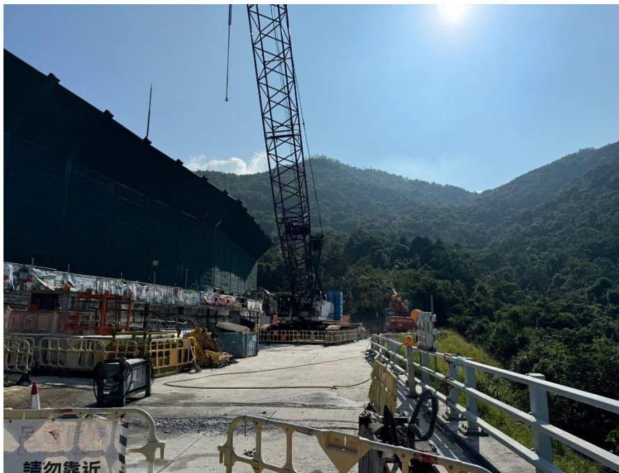
Photo B.10: Construction activities observed during the monitoring on 22 October 2024 but not adjacent to the receptor site.
