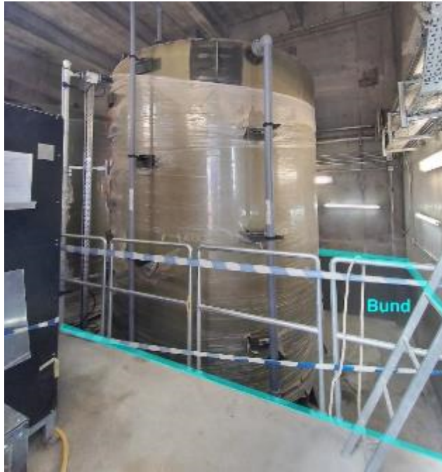
Ferric Chloride Storage Bund
