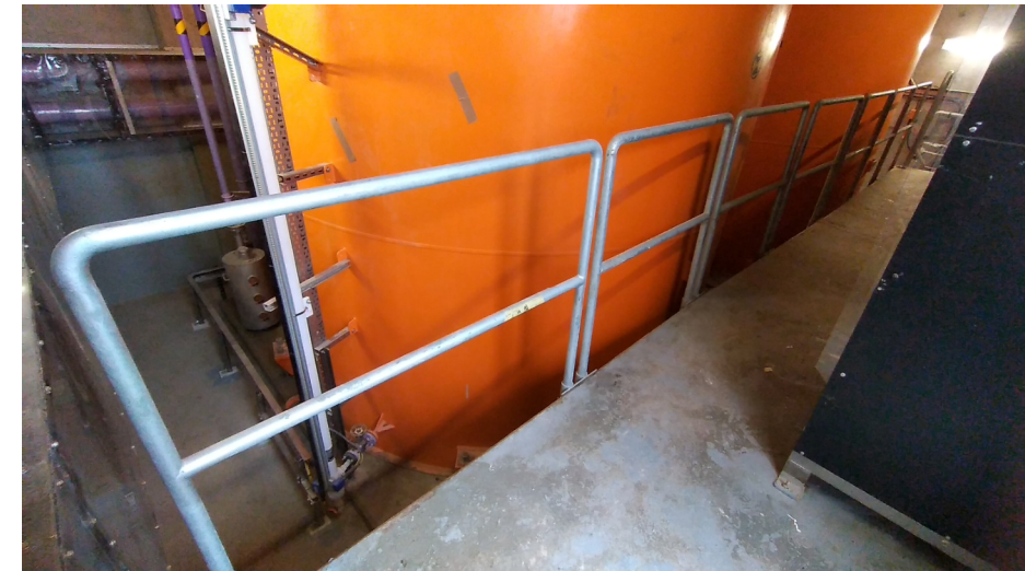
Sulphuric Acid Storage Bund
