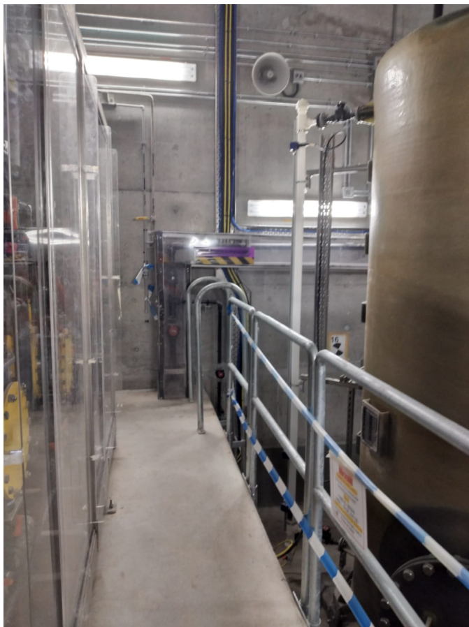
Hypochlorite Storage Bund
