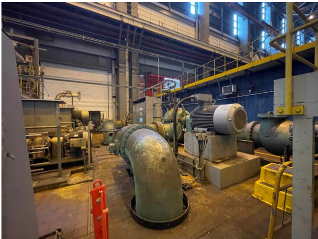
Photo 46: Other auxiliary system at the CPA Station Building
