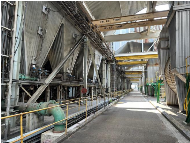
Photo 52: Electrostatic precipitator systems and induced draft fans
