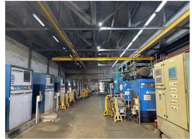
Photo 75: A compressor plant house with a series of compressors and blowers
