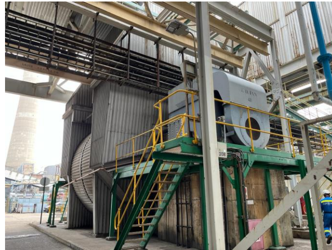
Photo 56: Induced draft fan of unit A4
