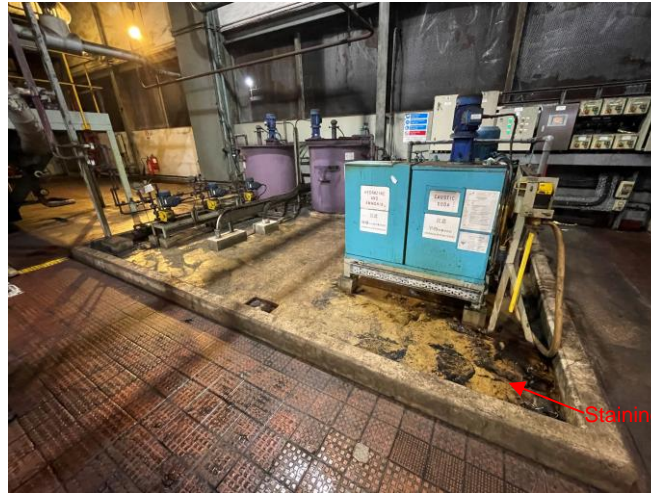
Photo 11: Chemical dosing system of unit A3 at turbine house
