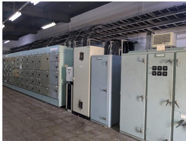
Photo 77: Ash plant substation
