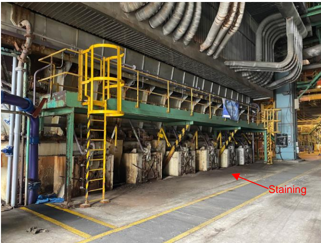
Photo 4: Ash hopper for furnace bottom ash at unit A4 inside boiler house
