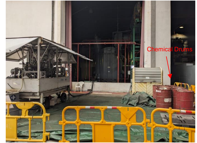
Photo 27: Generator transformer of unit A4 and maintenance area
