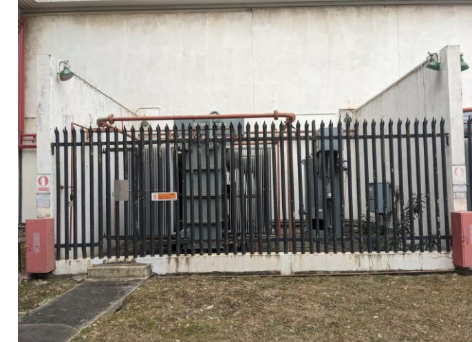
Photo 30: Unit auxiliary transformer of unit A2
