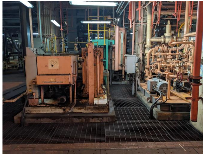
Photo 14: Seal oil system and lubrication oil system located at the drain sump
