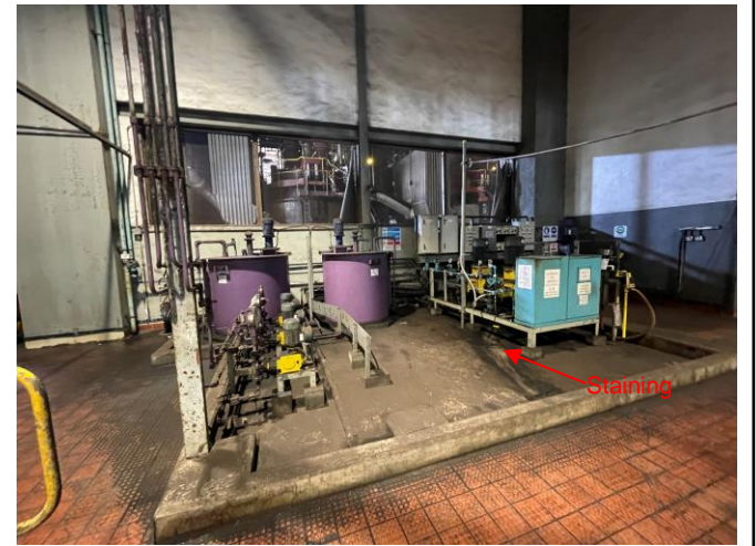
Photo 12: Chemical dosing system of unit A4 at turbine house
