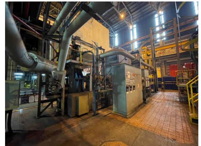
Photo 45: Other auxiliary system at the CPA Station Building
