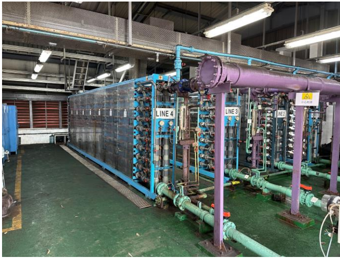
Photo 91: An electrochlorination plant house
