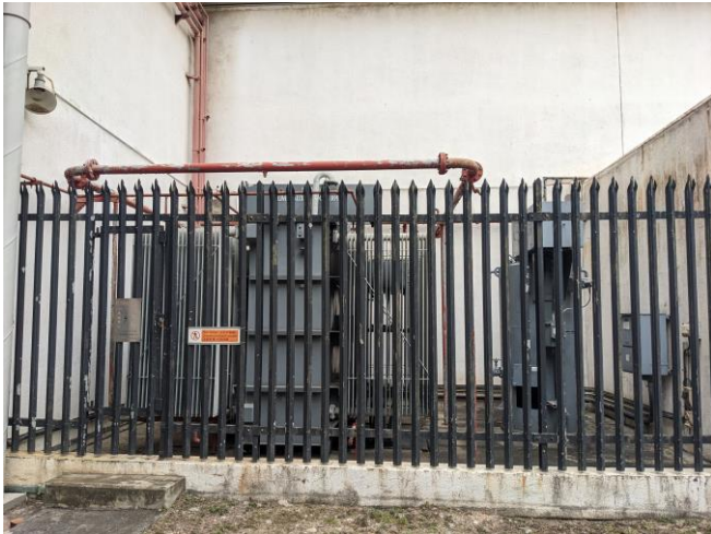
Photo 34: Unit auxiliary transformer of unit A4
