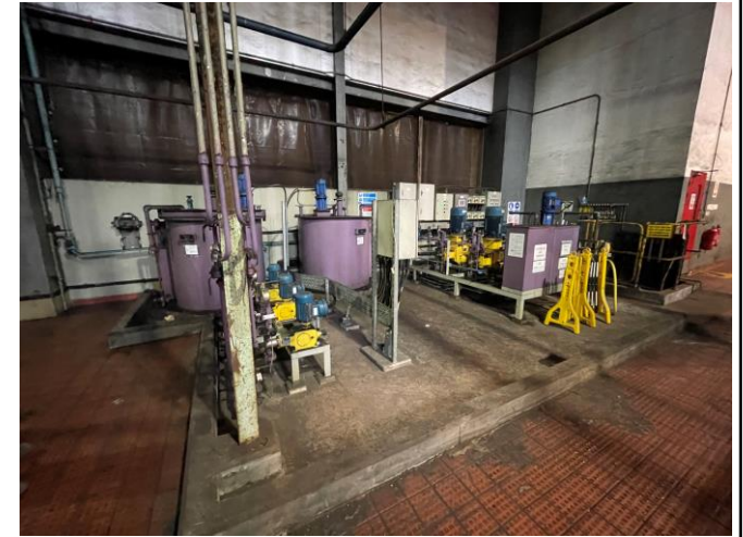
Photo 9: Chemical dosing system of unit A1 at turbine house
