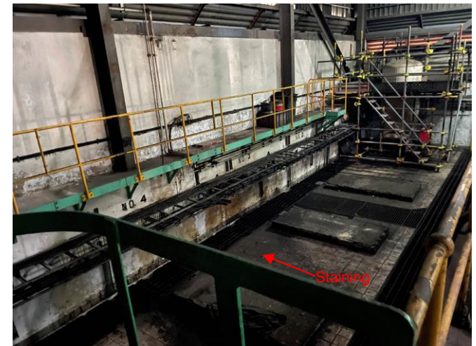
Photo 84: Fuel oil pump house
