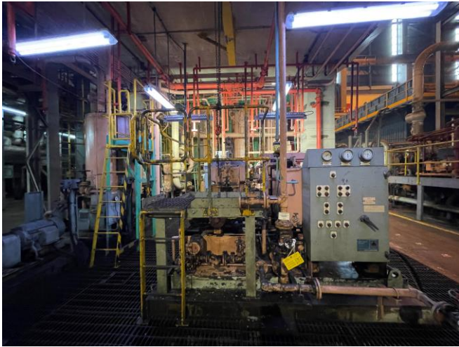
Photo 13: Seal oil system and lubrication oil system at unit A1
