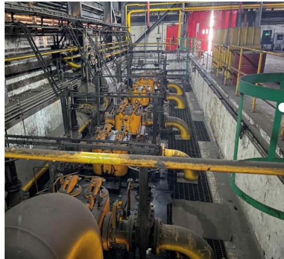
Photo 83: Fuel oil heaters in the fuel oil pump house
