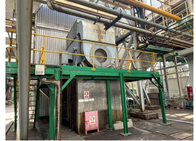
Photo 57: Induced draft fan of unit A1
