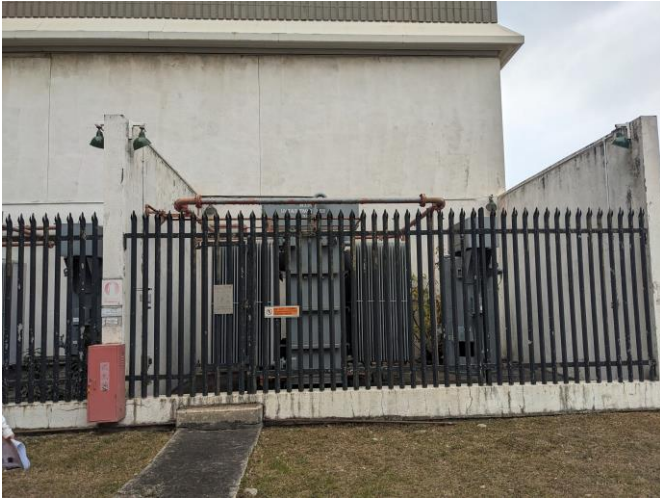
Photo 31: Unit auxiliary transformer of unit A2
