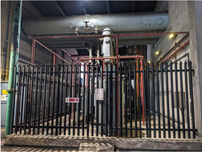
Photo 37: Unit transformer of unit A3
