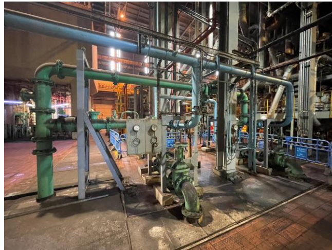
Photo 47: Other auxiliary system at the CPA Station Building
