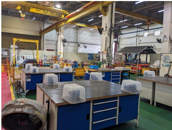
Photo 64: A training workshop area in the control block, workshop and store building
