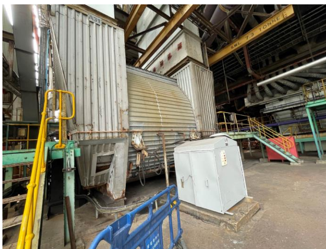
Photo 23: Forced draft fans of unit A2
