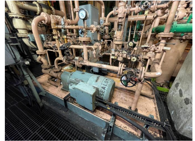
Photo 15: A seal oil unit
