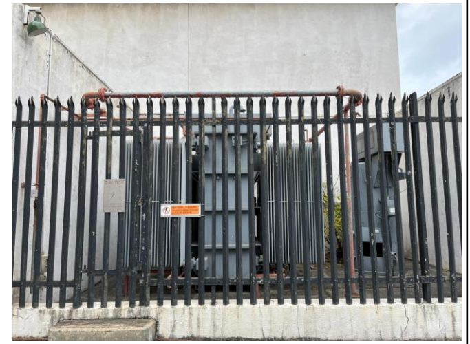
Photo 33: Unit auxiliary transformer of unit A3
