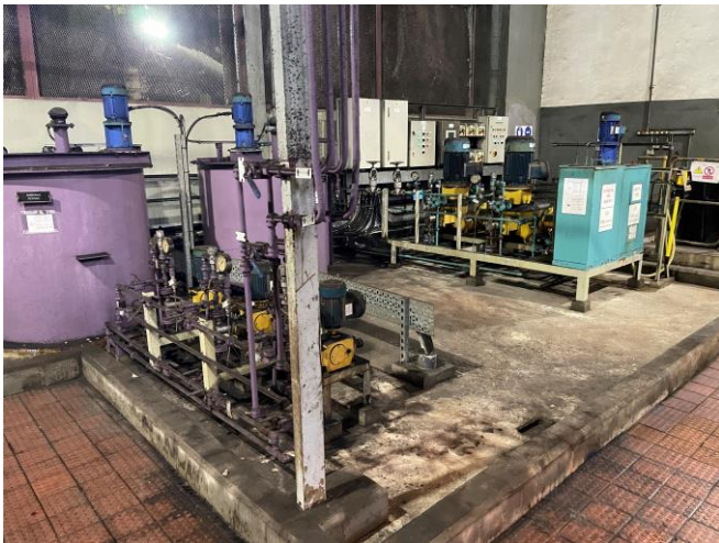
Photo 10: Chemical dosing system of unit A2 at turbine house
