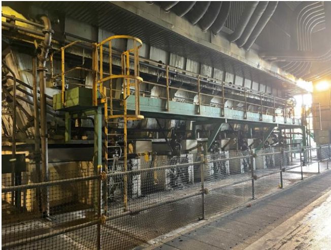
Photo 1: Ash hopper for furnace bottom ash at unit A1 inside boiler house
