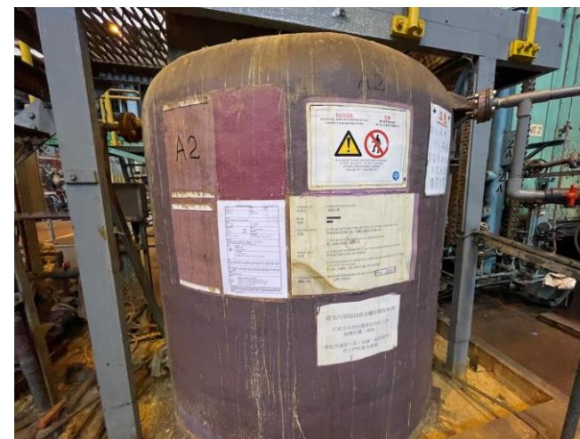
Photo 21: Ferrous sulphate tanks
