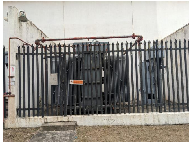
Photo 35: Unit auxiliary transformer of unit A4
