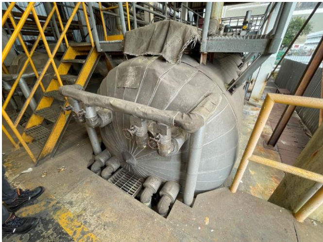
Photo 88: Sulphur melting tanks next to the sulfur store
