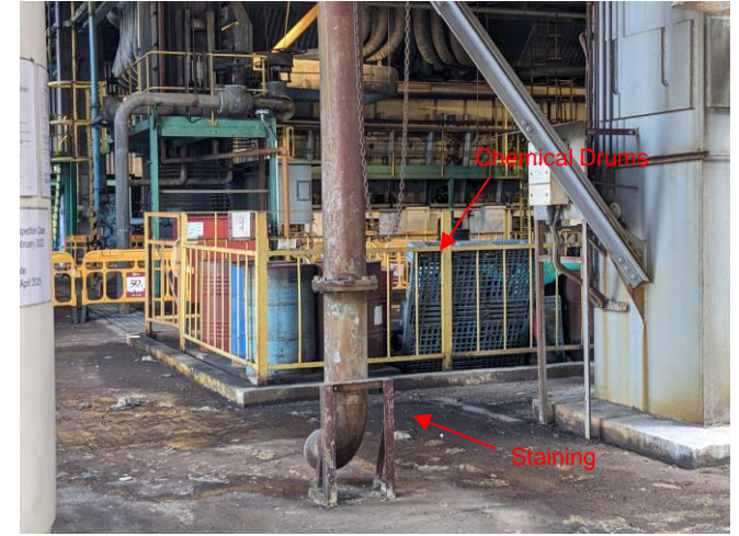
Photo 51: A chemical drum storage area was observed at unit A1 in the boiler house
