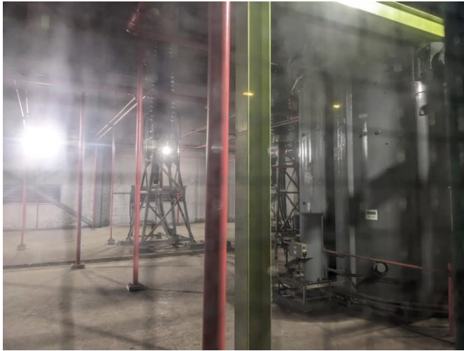
Photo 25: Generator transformer of unit A1
