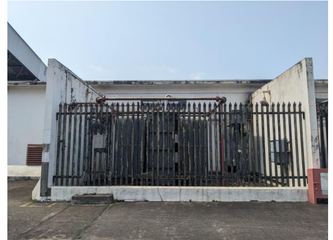
Photo 39: Station auxiliary transformer at ash plant
