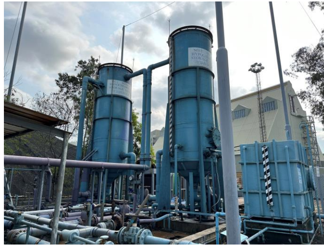
Photo 92: Two (2) aboveground tanks for storing sodium hypochlorite solution
