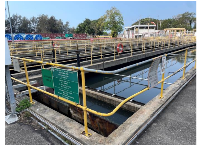
Photo 72: Oil separator system
