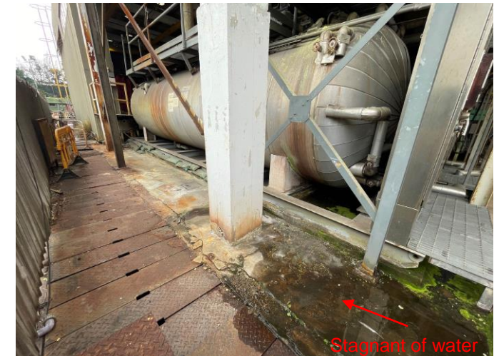
Photo 90: Sulphur melting tanks next to the sulfur store
