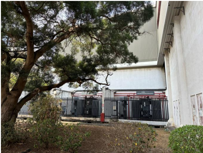
Photo 28: Station stand-by transformer and unit auxiliary transformer of unit A1
