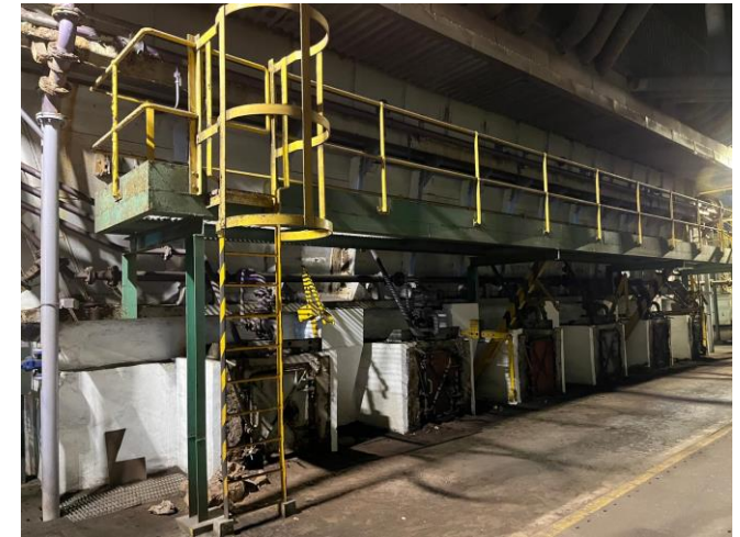
Photo 3: Ash hopper for furnace bottom ash at unit A3 inside boiler house
