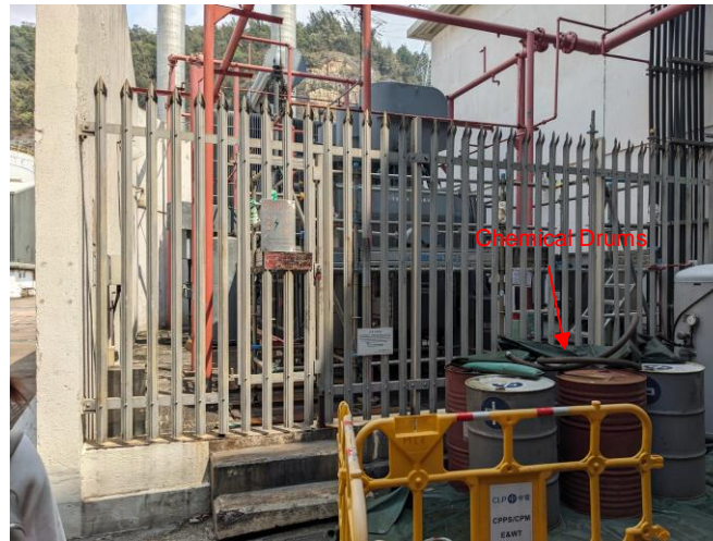
Photo 29: Station transformer and transformer maintenance area of unit A2
