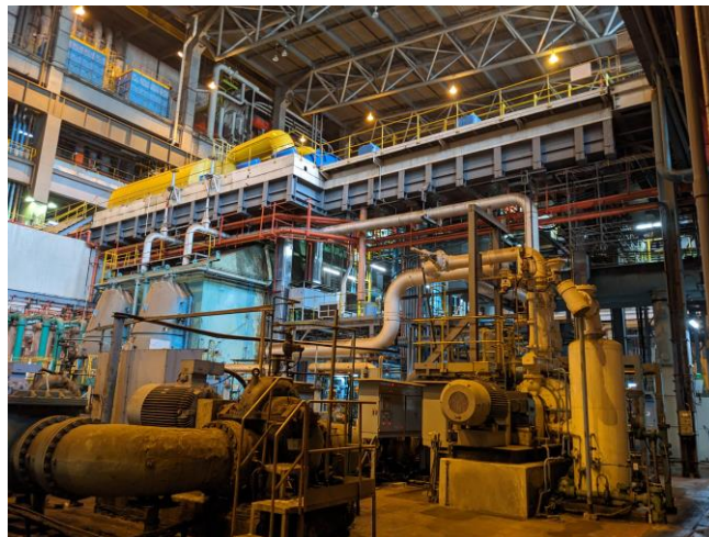
Photo 44: Other auxiliary system at the CPA Station Building
