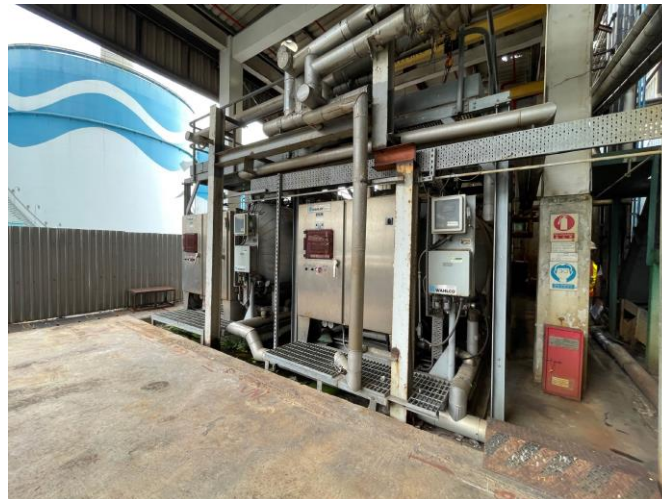
Photo 89: Sulphur melting tanks next to the sulfur store
