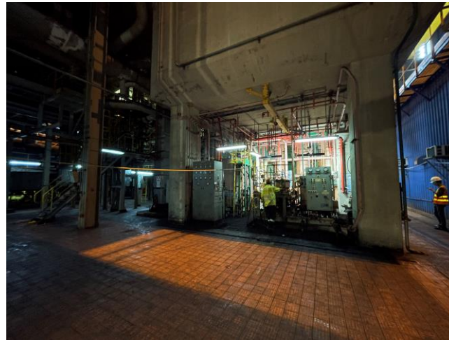
Photo 17: Seal oil system and lubrication oil system at unit A1
