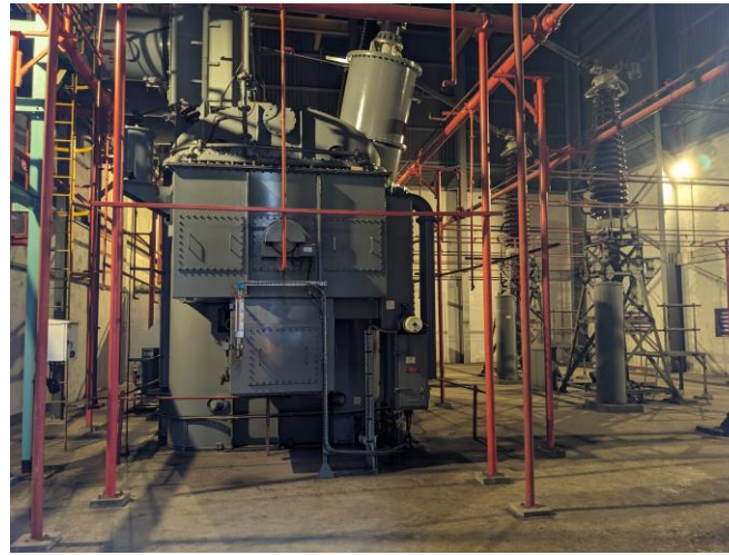
Photo 26: Generator transformer of unit A3
