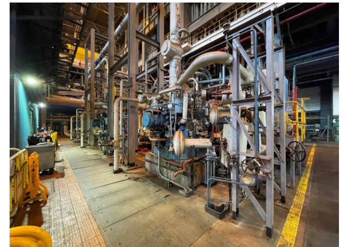
Photo 48: Other auxiliary system at the CPA Station Building
