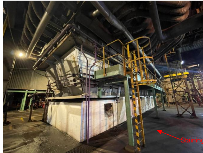
Photo 2: Ash hopper for furnace bottom ash at unit A2 inside boiler house
