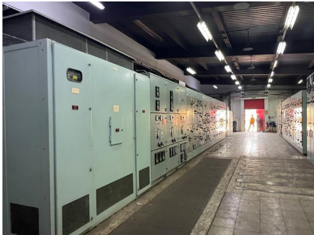
Photo 76: Ash plant substation
