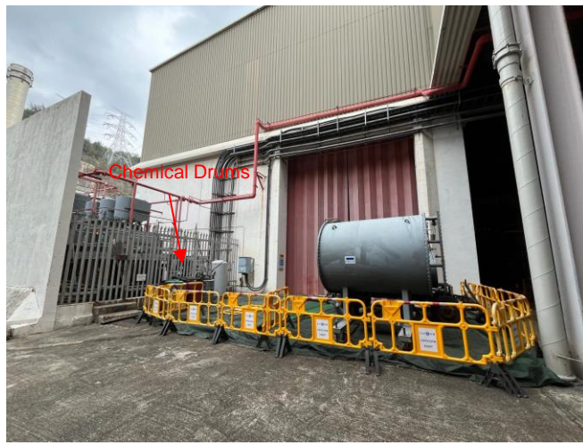
Photo 41: Transformer maintenance area at units A2
