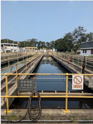
Photo 73: Oil separator system
