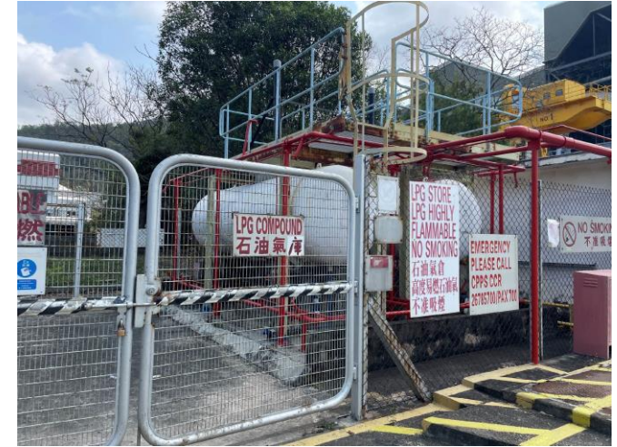
Photo 81: Liquefied Petroleum Gas (LPG) Store
