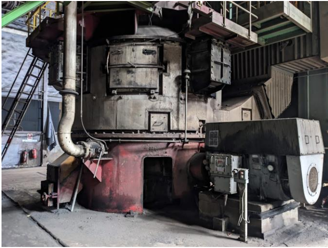
Photo 7: A coal grinding mill at unit A4
