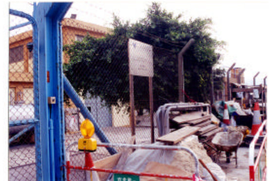
3 SALT WATER PUMPING STATION
