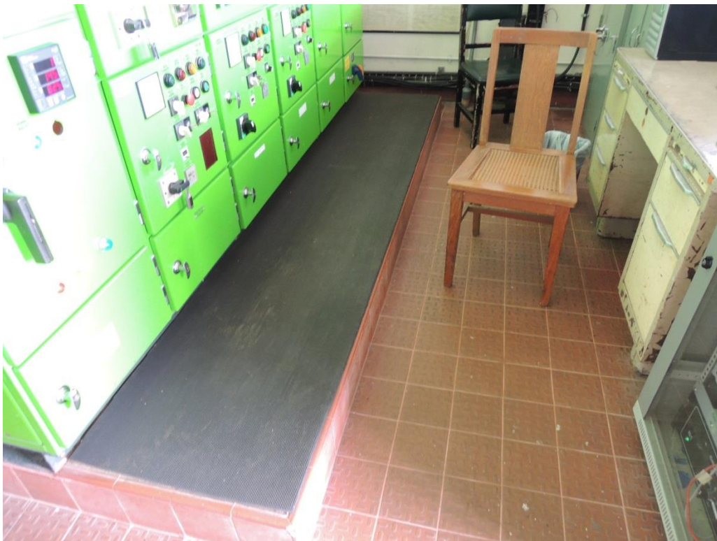
Photo 10 - Control Room of the Existing Sha Tau Kok Sewage Treatment Works (Interior View)
