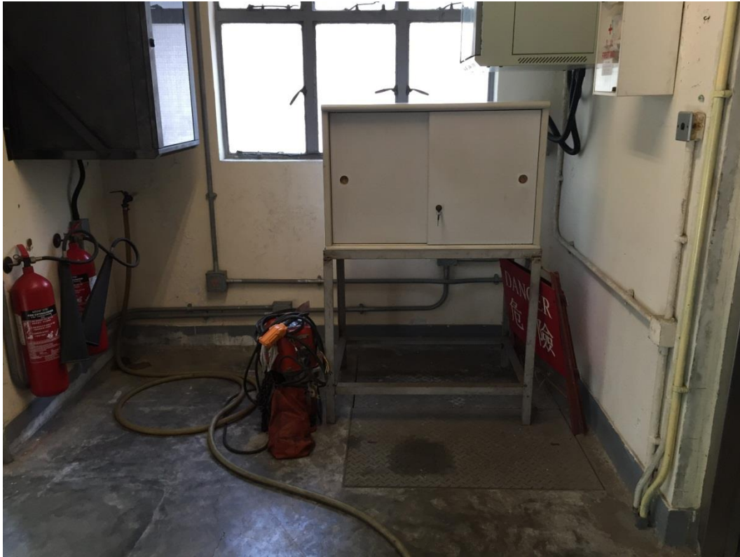
Photo 3 - Existing Sha Tau Kok Sewage Pumping Station at Shun Hing Street (Interior View)
