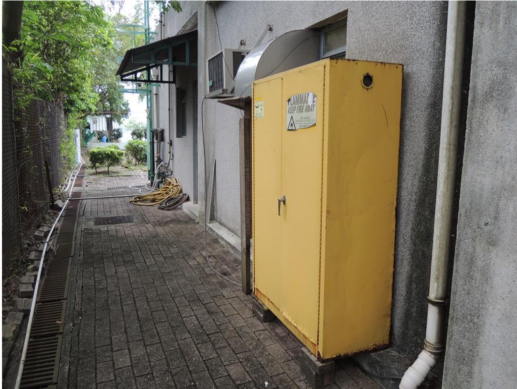
Photo 11 - Chemical Storage Cabinet in the Existing Sha Tau Kok Sewage Treatment Works
