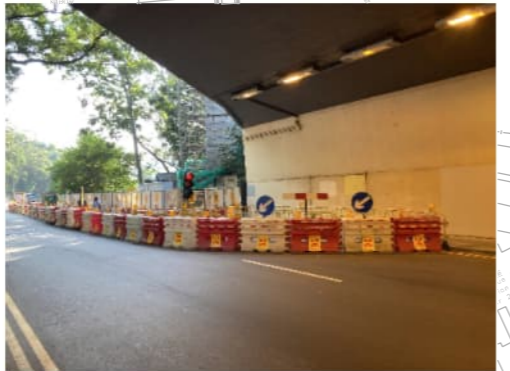
PHOTO 1088: WING SHUN STREET AND WORKS AREA OF CONTRACT HY/2016/02 (DATE TAKEN: 16 NOVEMBER 2021)
