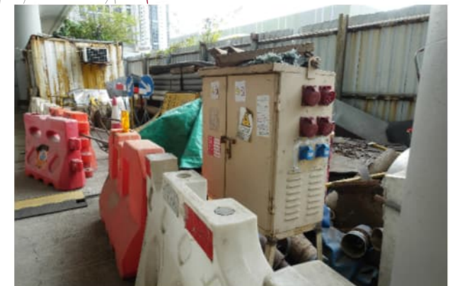
PHOTO 9032: ELECTRICITY SUPPLY (DATE TAKEN: 22 DECEMBER 2021)
