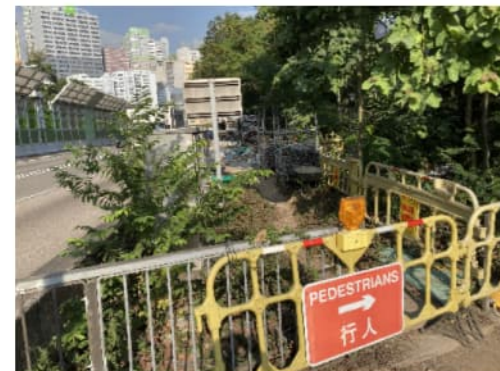
PHOTO 1100: WORKS SITE OF CONTRACT NO. HY/2016/02 AND TSING TSUEN ROAD (DATE TAKEN: 16 NOVEMBER 2021)
