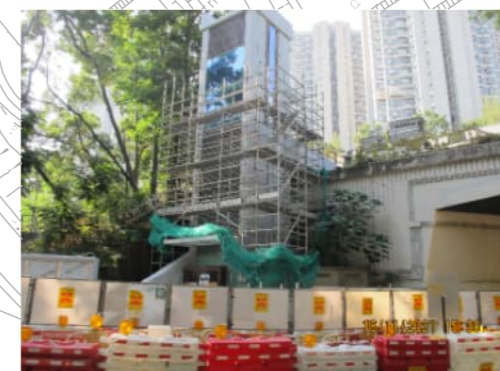
PHOTO 9043: WORKS SITE OF CONTRACT NO. HY/2016/02 AND TSING TSUEN ROAD (DATE TAKEN: 16 NOVEMBER 2021)
