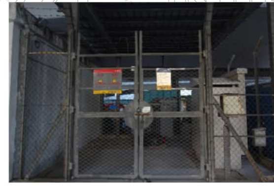
PHOTO 8679: TRANSFORMER OF TSUEN WAN REGIONAL LABORATORY SUBSTATION (TO BE RETAINED) (DATE TAKEN: 16 NOVEMBER 2021)
