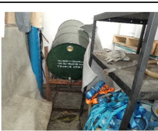
PHOTO 5063: MOTOR OIL STORAGE (DATE TAKEN: 22 DECEMBER 2021)
