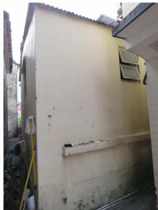
Side view of HB-22, showing southeast and northeast facing elevations, looking northwest.
