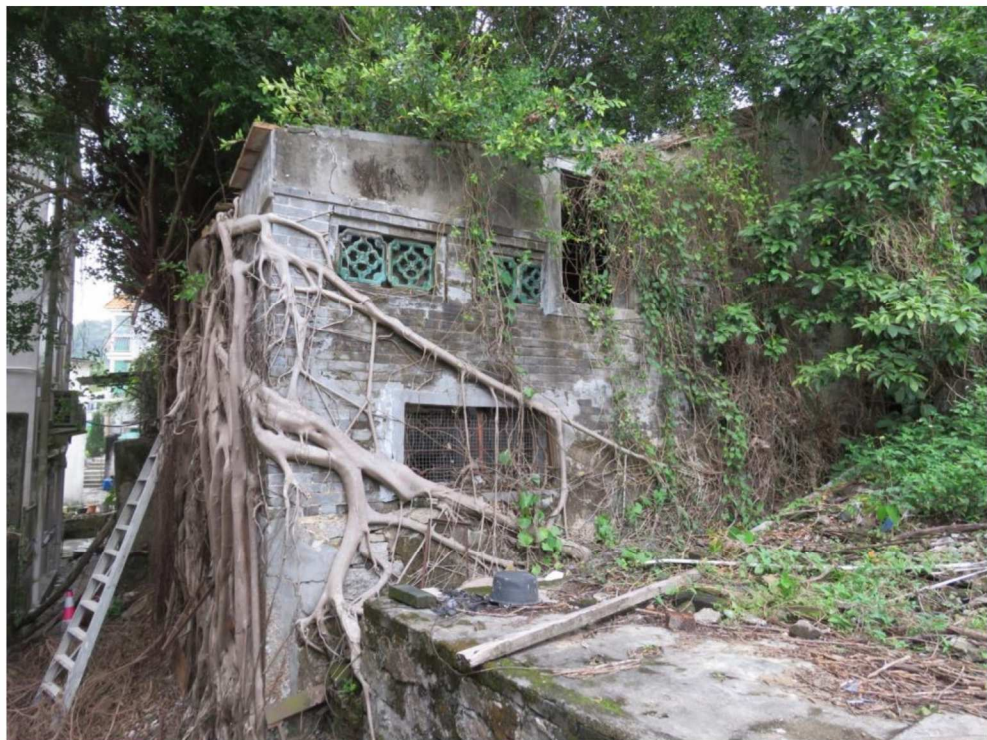
General view of HB-15, showing southwest and southeast facing elevations, looking west.
