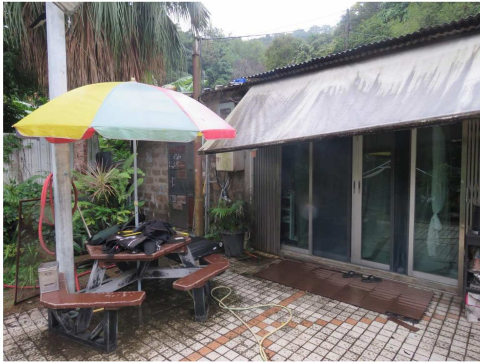
Close-in view of southern façade, showing masonry structure at the end, looking southwest.
