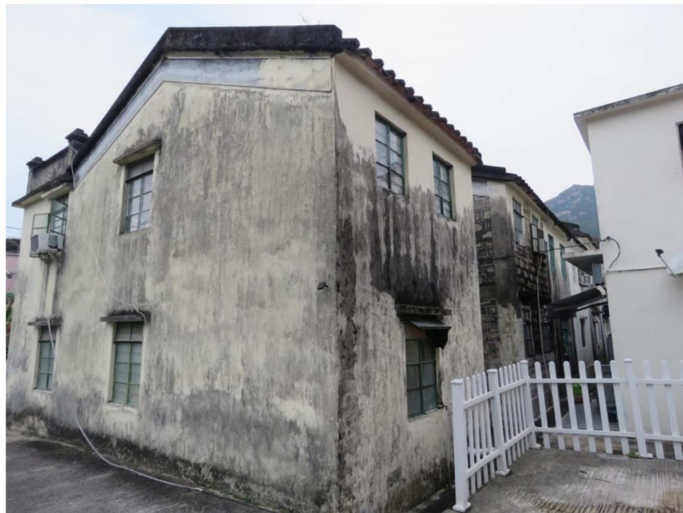
Side and rear view of HB-07, showing southeast and northeast elevations, looking northwest.
