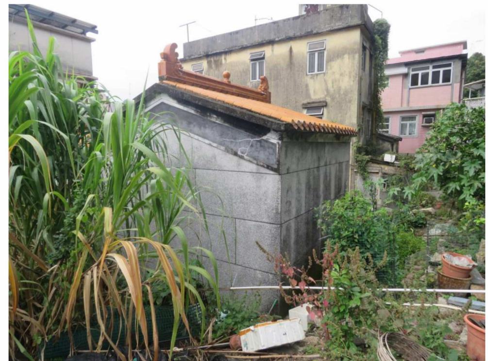
Side and rear view of HB-03, showing southeast and northeast elevations, looking west.
