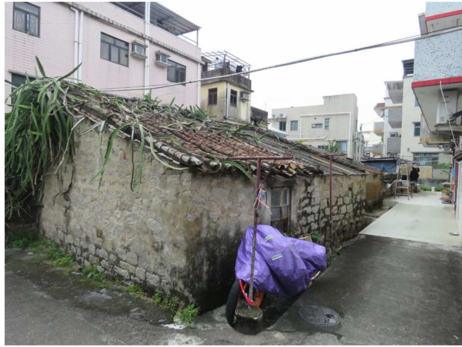
Side and rear view of HB-11, showing southeast and northeast facing elevations, looking southwest.
