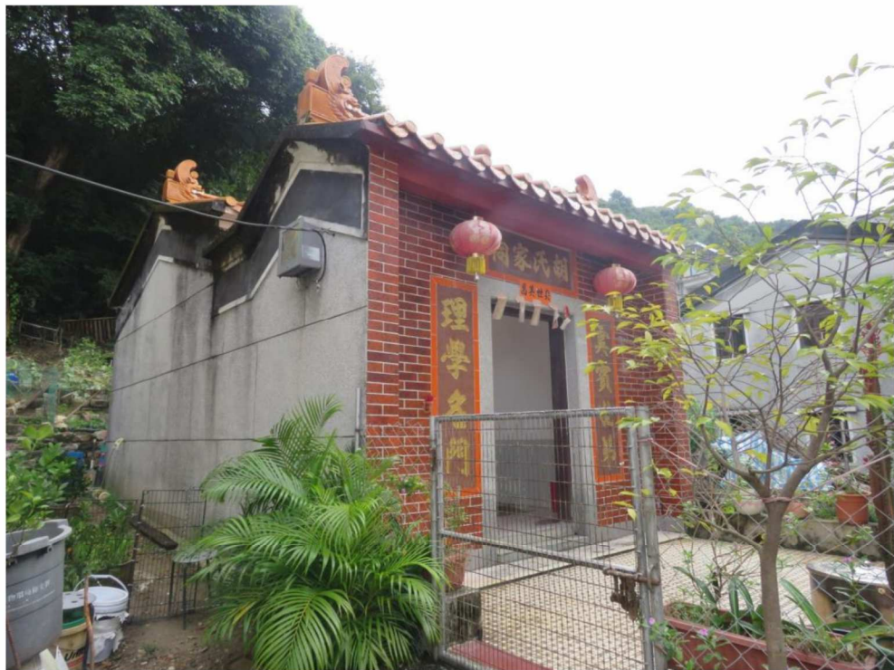
Façade and side view of HB-03, showing northwest and southwest facing elevations, looking east.
