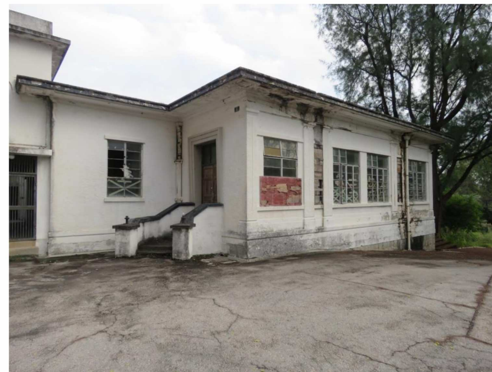
Front and side view of GB-01, showing entrance and west facing elevations, looking southeast.
