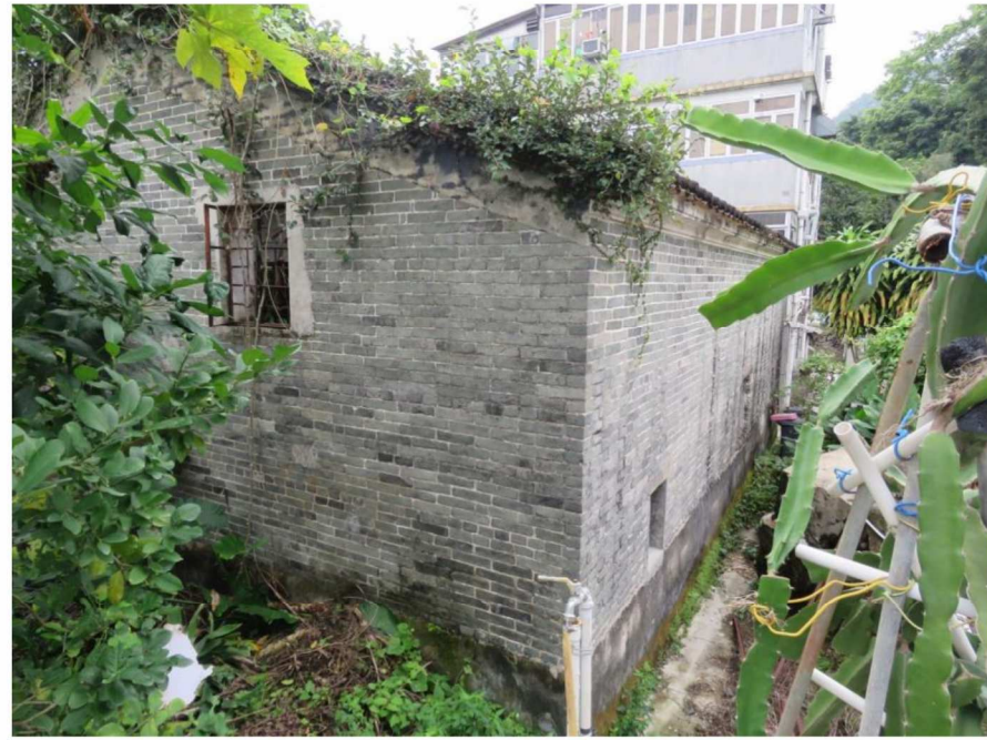
Side and rear view of GB-04, showing rear part of southeast facing and northeast facing elevations, looking southwest.
