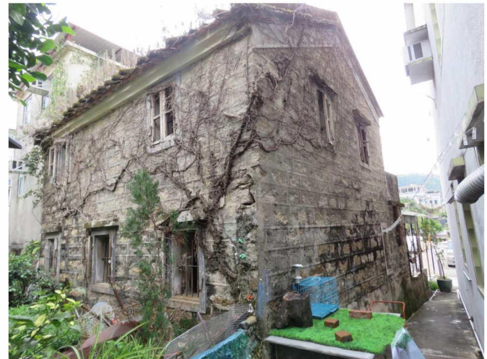
Rear and side view of HB-18, showing north and west elevations, looking southeast.
