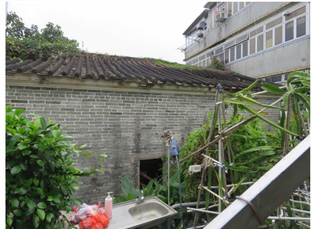
Rear view of GB-04, showing northeast facing elevation and deformed roof, looking southwest.
