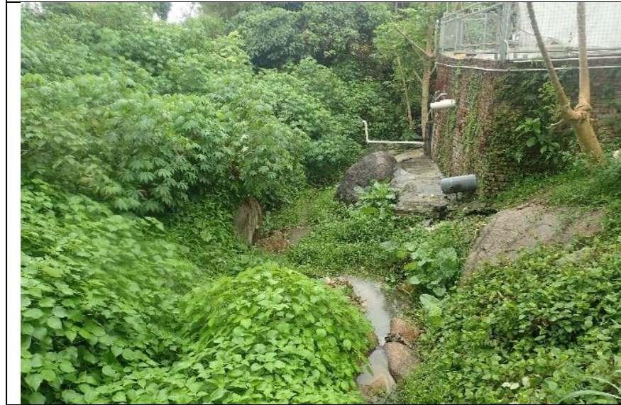
The ditch falling within the aboveground works area in So Kwun Wat
