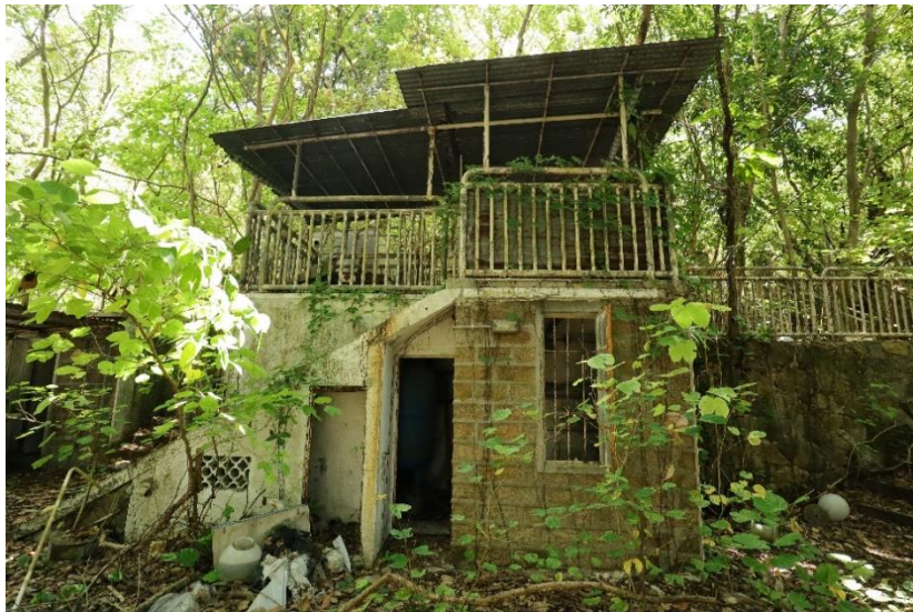
3- Utilities Control Room
