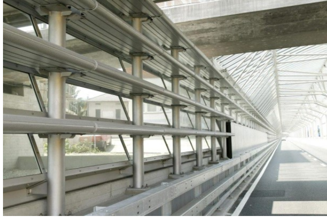
Angled noise barrier panel 1
