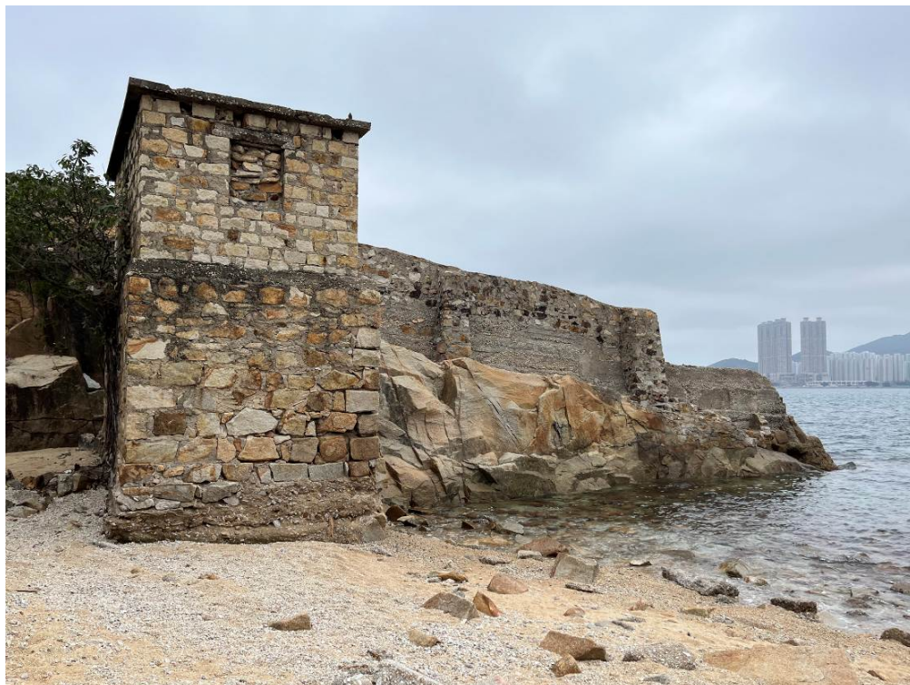
Plate 2.39. Western elevation of the stone hut in the east of the site, which was probably served as a dangerous goods store.
