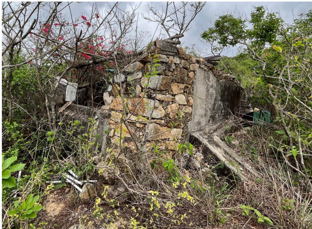
Plate 12.2. Exterior of the Pillbox which located to the east of Pottinger Battery (BH04).
