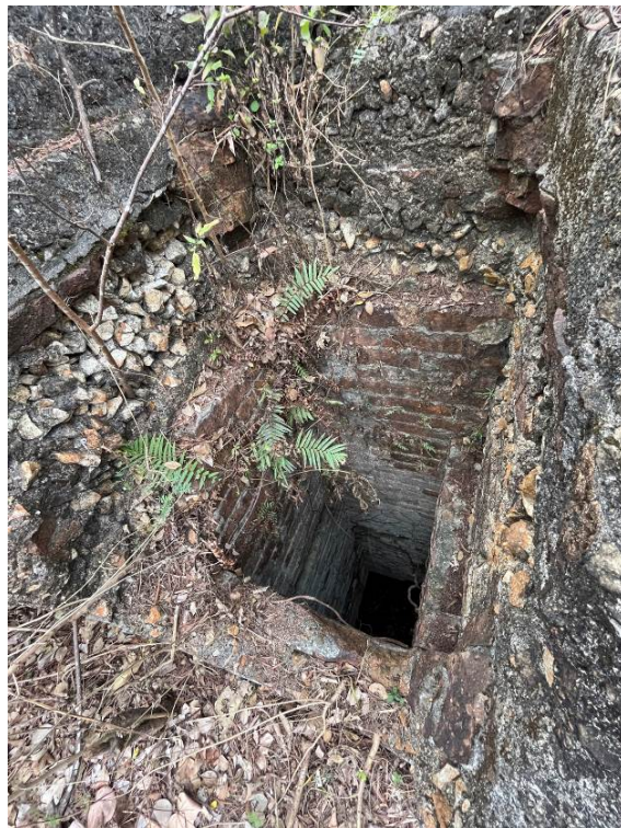
Plate 1.14. Vertical shaft, constructed of red bricks and concrete, connects the underground storage to the surface of the gun emplacement.
