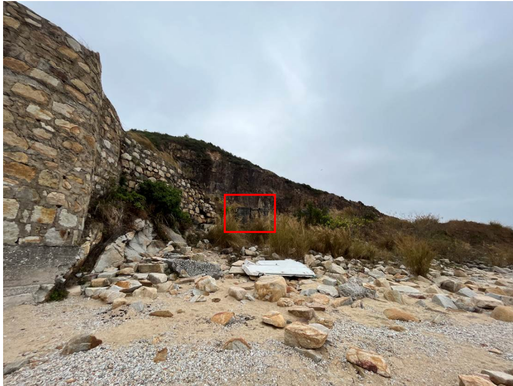
Plate 2.44. Concrete base for a stone crushing plant, situated on the edge of an artificial slope.
