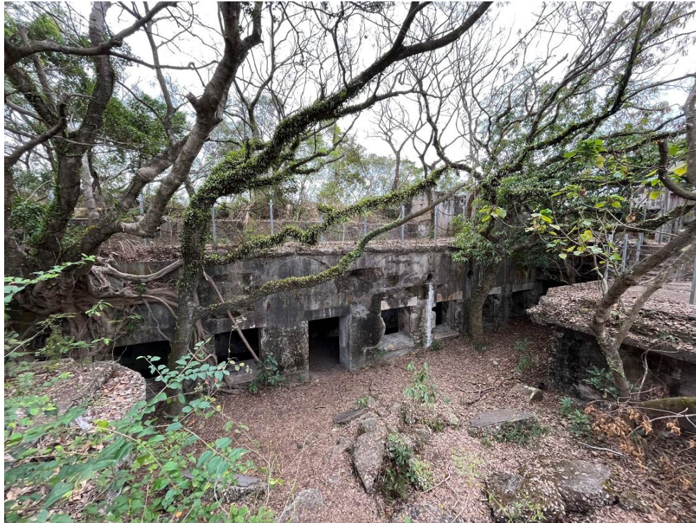
Plate 1.15. Underground magazine of the Gough Battery, it is exposed due to collapse of the roof slabs.
