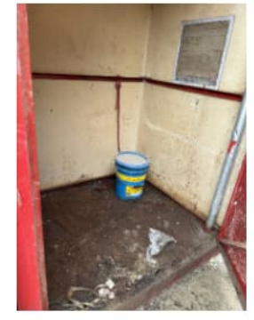
PHOTO 7510: CHEMICAL WASTE STORAGE CABINET DATE TAKEN: 19 FEBRUARY 2024
