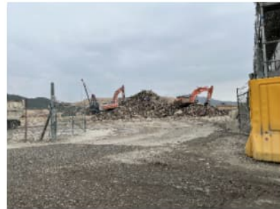
PHOTO 5432: BARGING POINT OF TSEUNG KWAN O AREA 137 CONSTRUCTION WASTE SORTING FACILITIES DATE TAKEN: 19 FEBRUARY 2024
