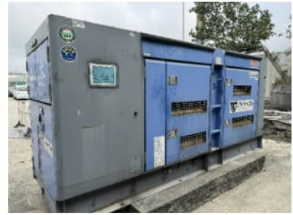
PHOTO 8320: GENERATOR DATE TAKEN: 22 FEBRUARY 2024
