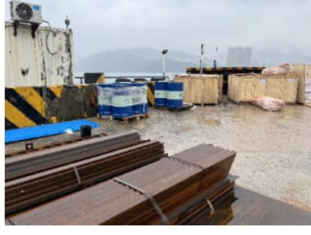
PHOTO 7027: CONSTRUCTION MATERIALS AND LUBRICANT GEAR OIL DRUMS STORAGE AREA DATE TAKEN: 11 MARCH 2024
