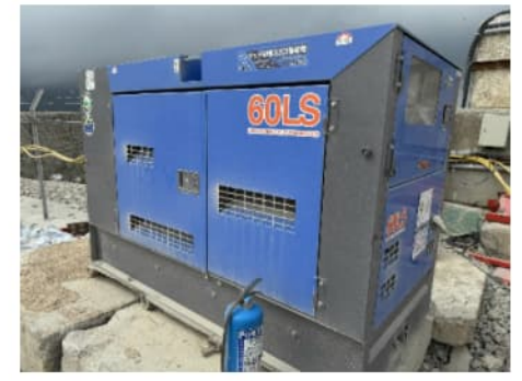
PHOTO 8341: GENERATOR DATE TAKEN: 22 FEBRUARY 2024
