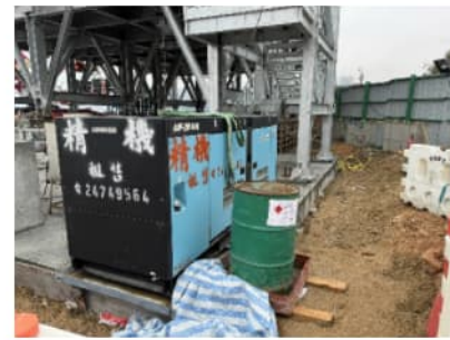
PHOTO 8776: DIESEL OIL DRUM AND GENERATOR DATE TAKEN: 11 MARCH 2024
