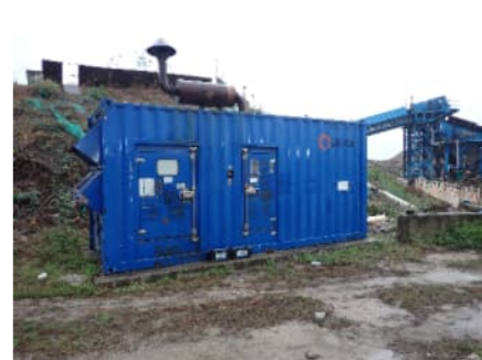
PHOTO 8608: GENERATOR DATE TAKEN: 11 MARCH 2024
