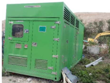
PHOTO 7859: GENERATOR DATE TAKEN: 19 FEBRUARY 2024
