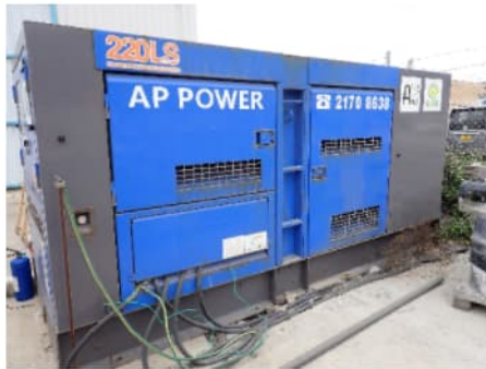
PHOTO 8174: GENERATOR DATE TAKEN: 22 FEBRUARY 2024
