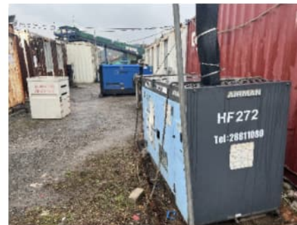
PHOTO 7013: GENERATORS DATE TAKEN: 11 MARCH 2024
