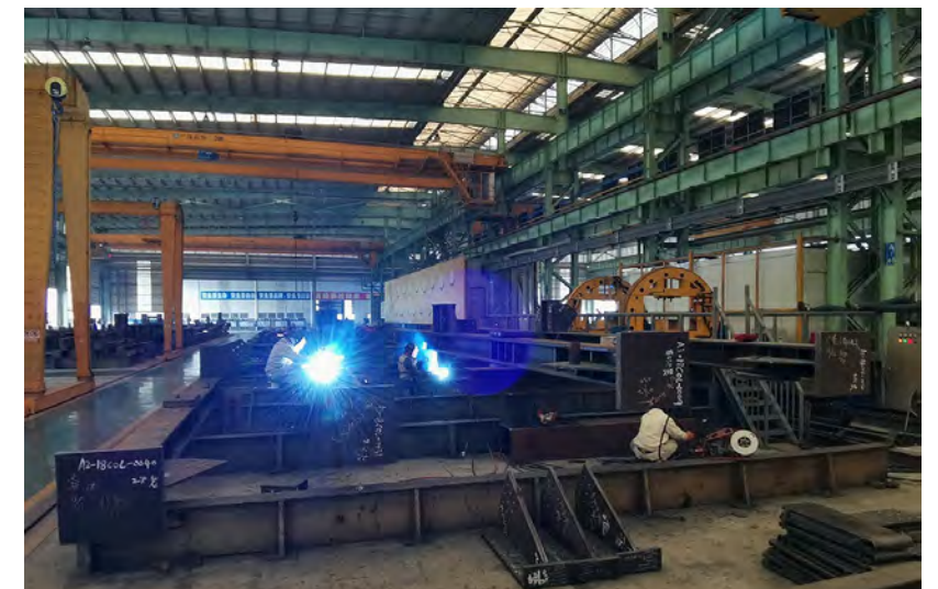
| Welding and erection of a steel frame for prefabricated electrical and mechanical units at I-PARK's Prefabrication Yard in Zhuhai (December 2020)
