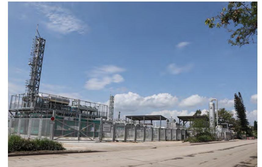
WENT Landfill Gas Power Generation Project
