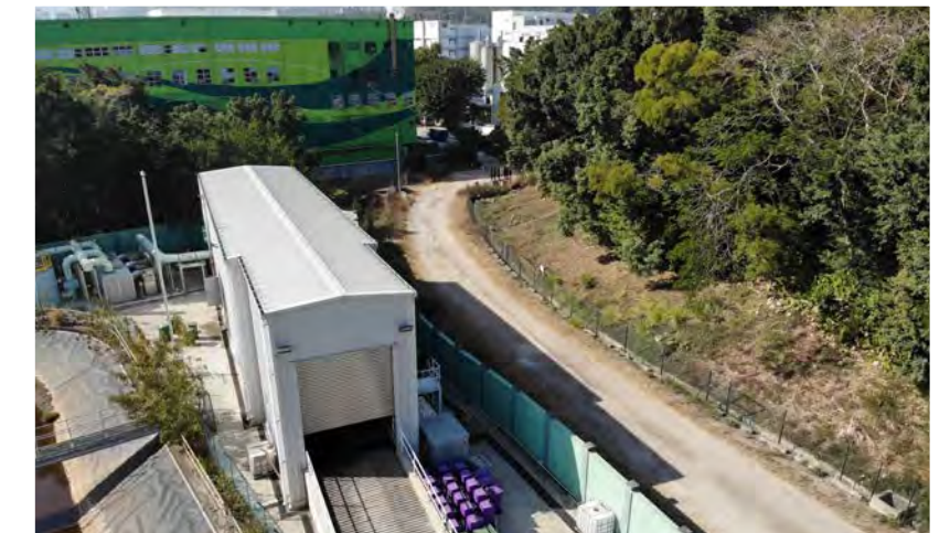
| Food Waste Pre-treatment Facilities for food waste/sewage sludge anaerobic co-digestion trial scheme at TPSTW
