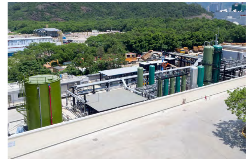
Landfill Gas Utilisation Plant at the SENT Landfill
